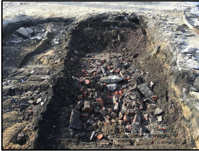
Photo 1: Brick Pile encountered at 20 Thames project
