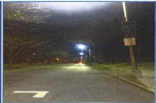
Baltimore After – LED Cobra Head Luminaires
