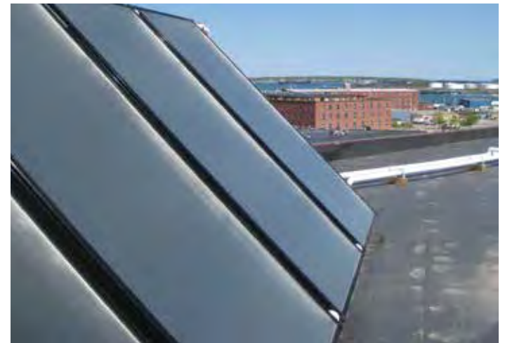
Above: 53 Danforth interior Bottom: Rooftop solar panels, 53 Danforth
