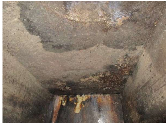
Concrete ceiling slab with minor infiltration
