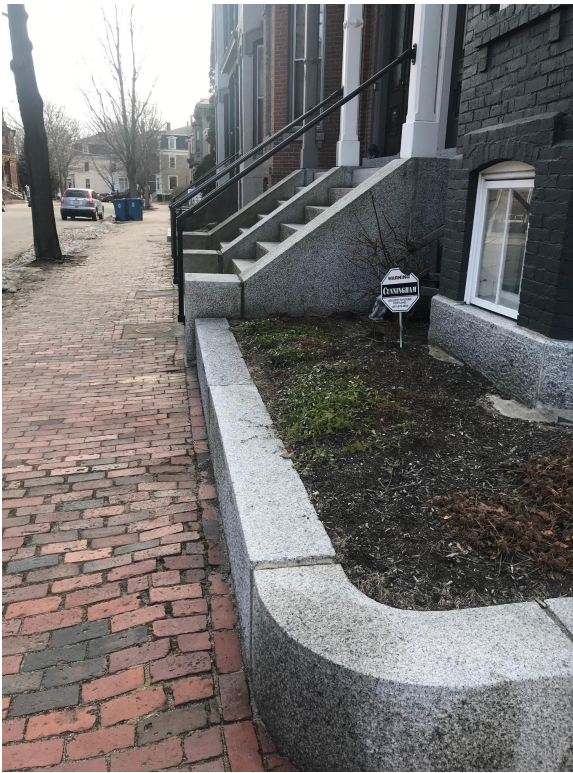
Residence at 144 Pine Street with a 10" W x 12" High granite curb wall. Retaining wall is needed to support soil for plant bed and prevent soil runoff onto sidewalk.
