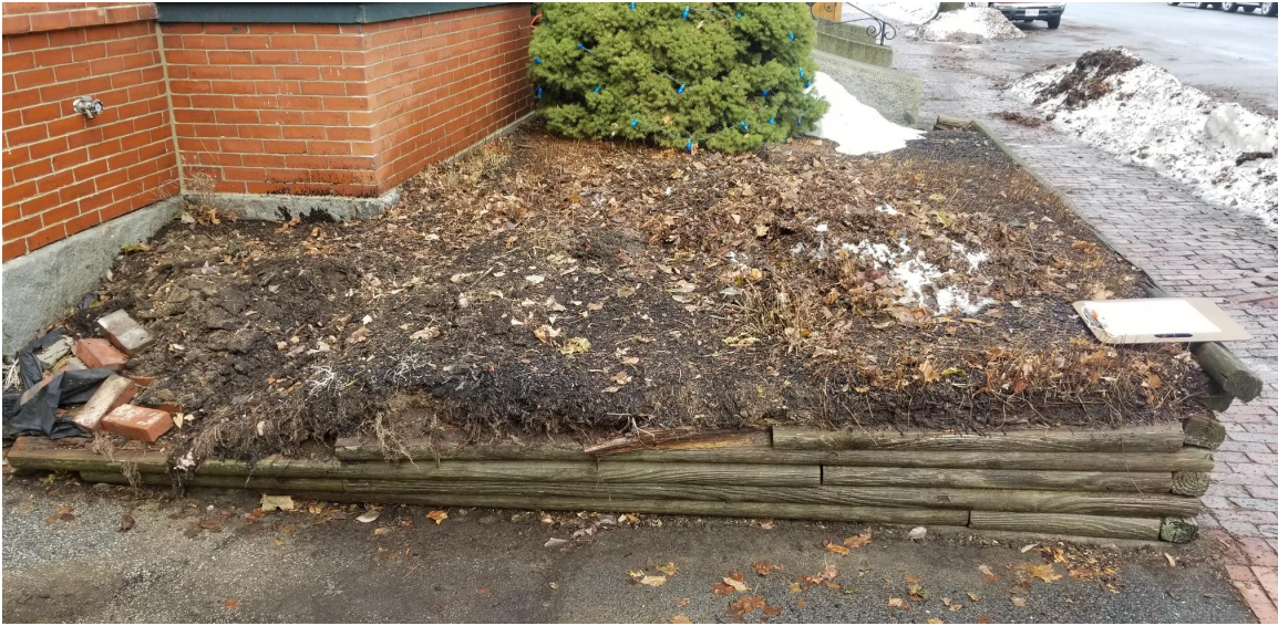
Existing condition of wooden timber retaining wall. Current wall slopes back into grade where it meets foundation of house. Wall is leaning towards driveway.
