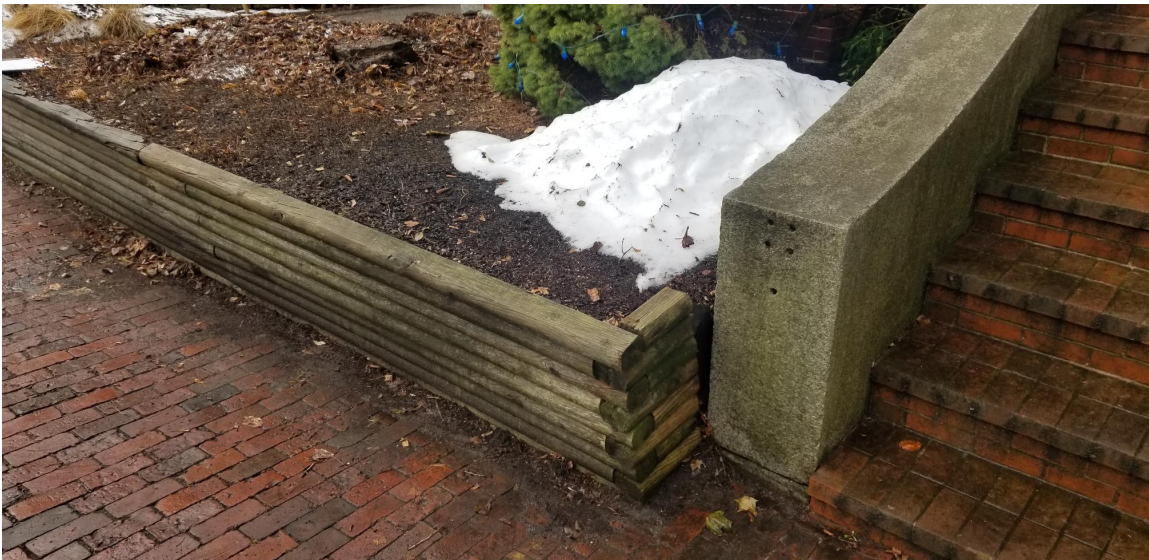
Existing view of corner of wooden timber retaining wall and concrete side wall of front steps. Timber retaining wall is leaning towards sidewalk.
