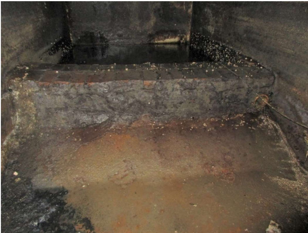
Figure 2-3: CSO 18 Regulator Structure Weir
