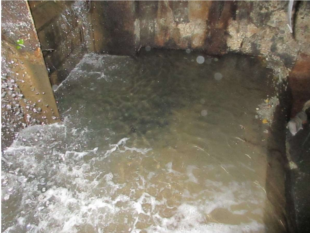
Figure 2-2: CSO 17 Regulator Structure Weir
