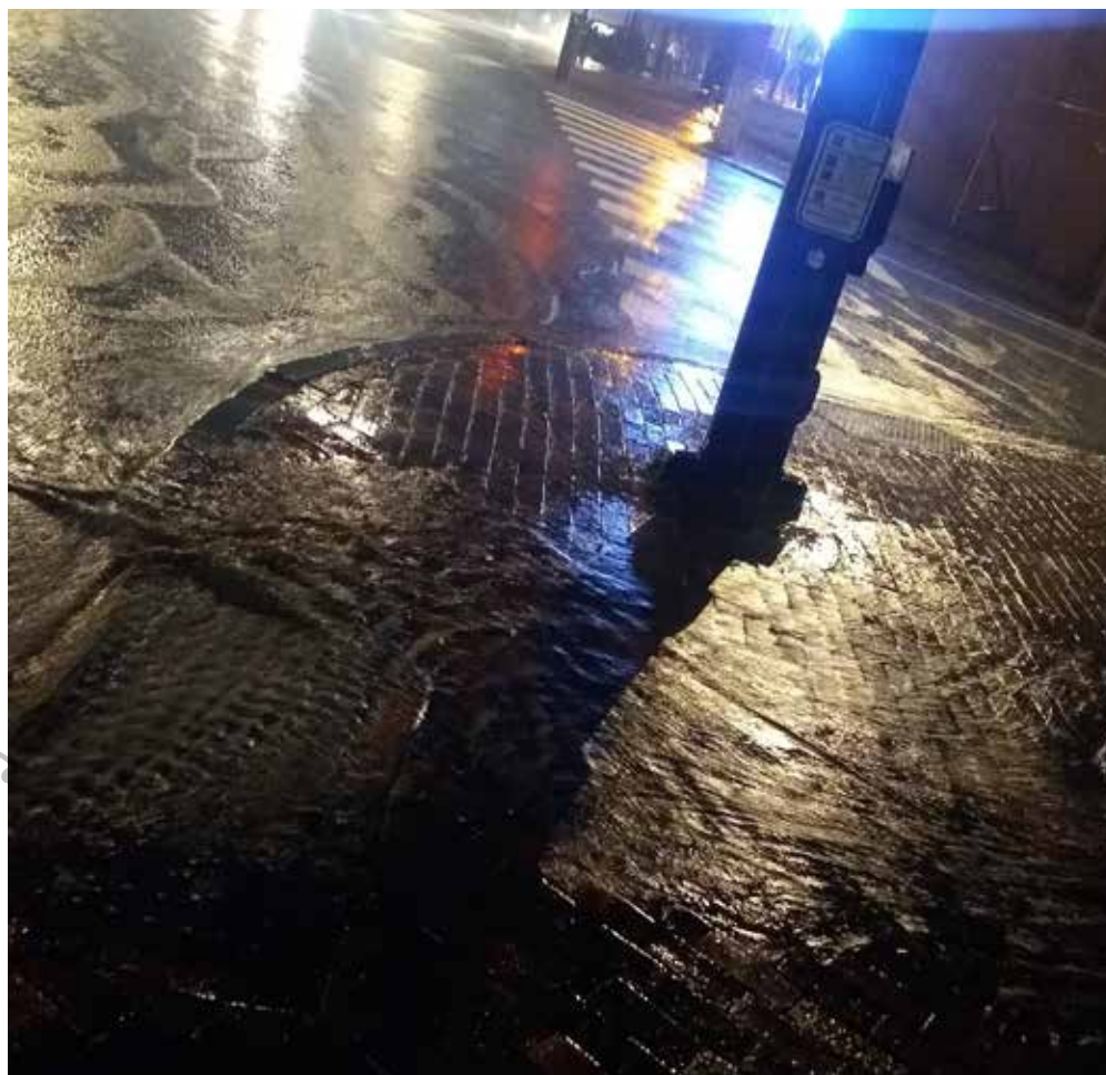
Curb ramp allows water to over-top sidewalk
