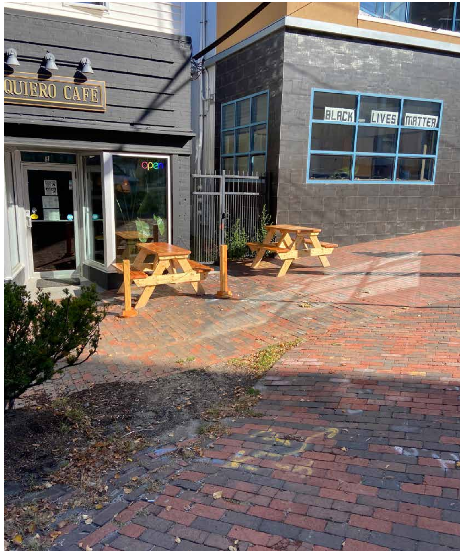
Accessibility and grading issues- existing condition does not provide a minimum 2% cross-slope
