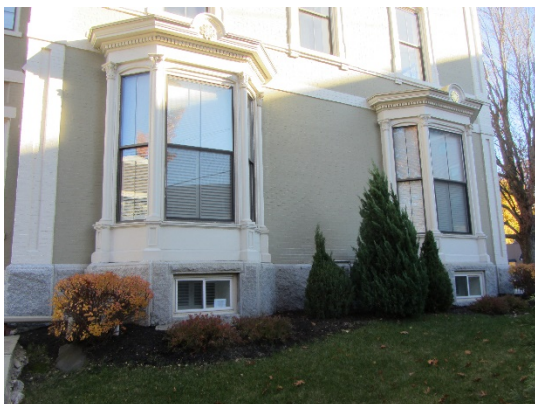
Heat pump installation – proposal called for installation high on wall between bays. Ground-mounting approved.
