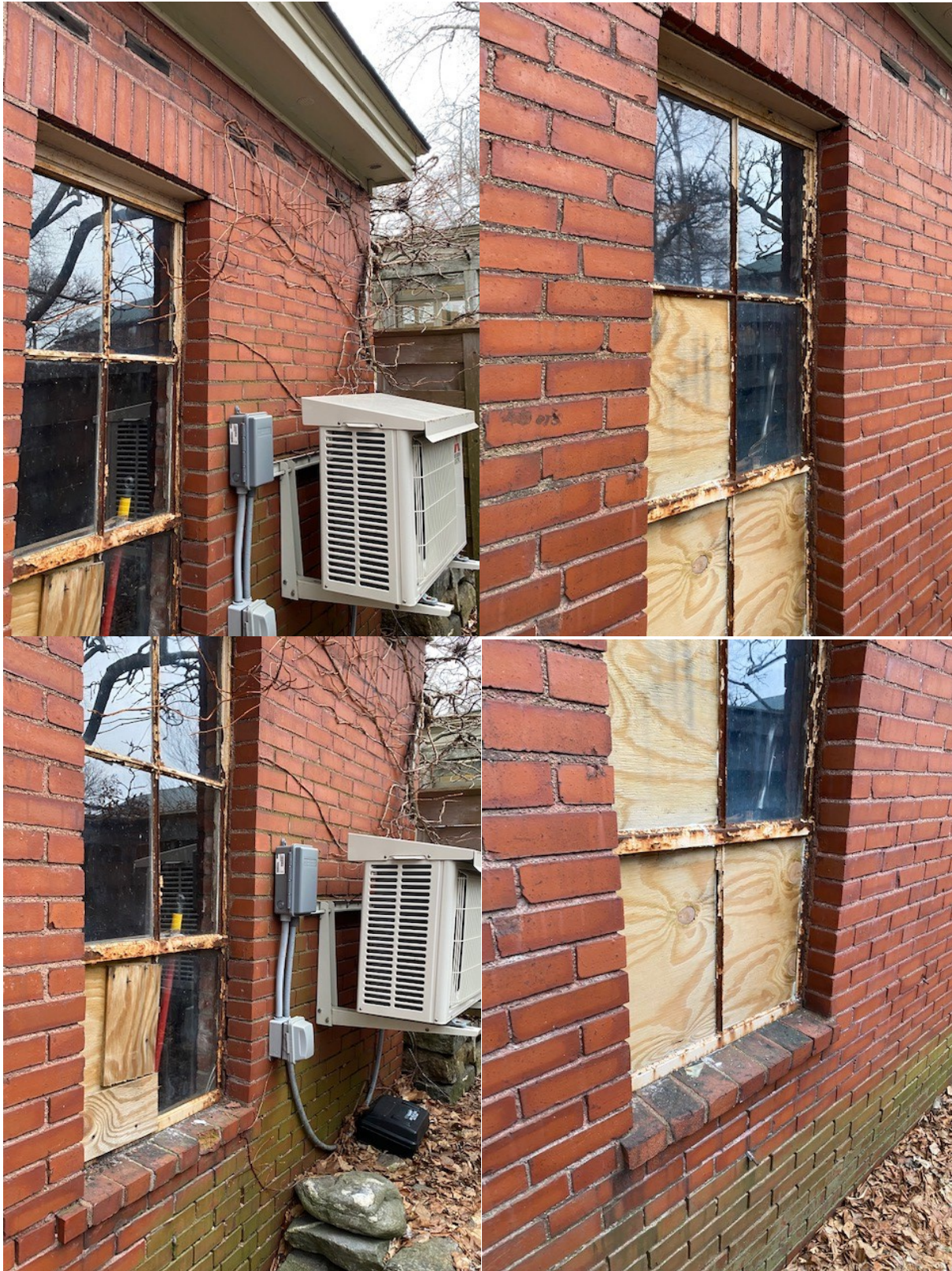
Close ups of each of the two steel windows and their poor condition.
