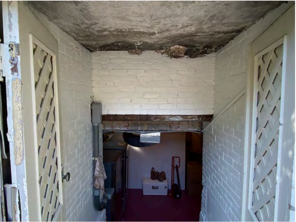
Closer view of obstructions
