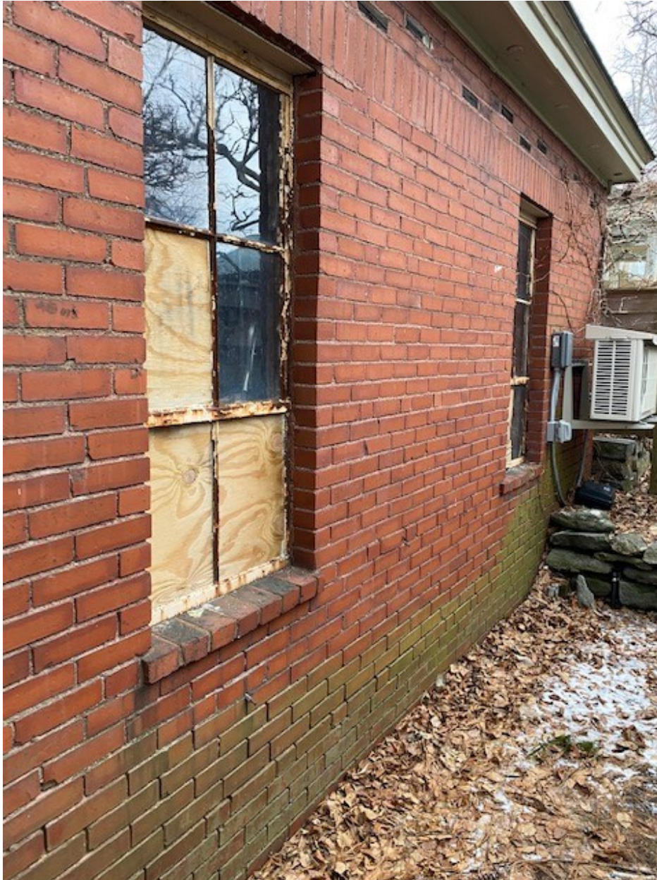
South side of the garage. Steel windows in poor condition. Mortar loss. Environmental dirt.
