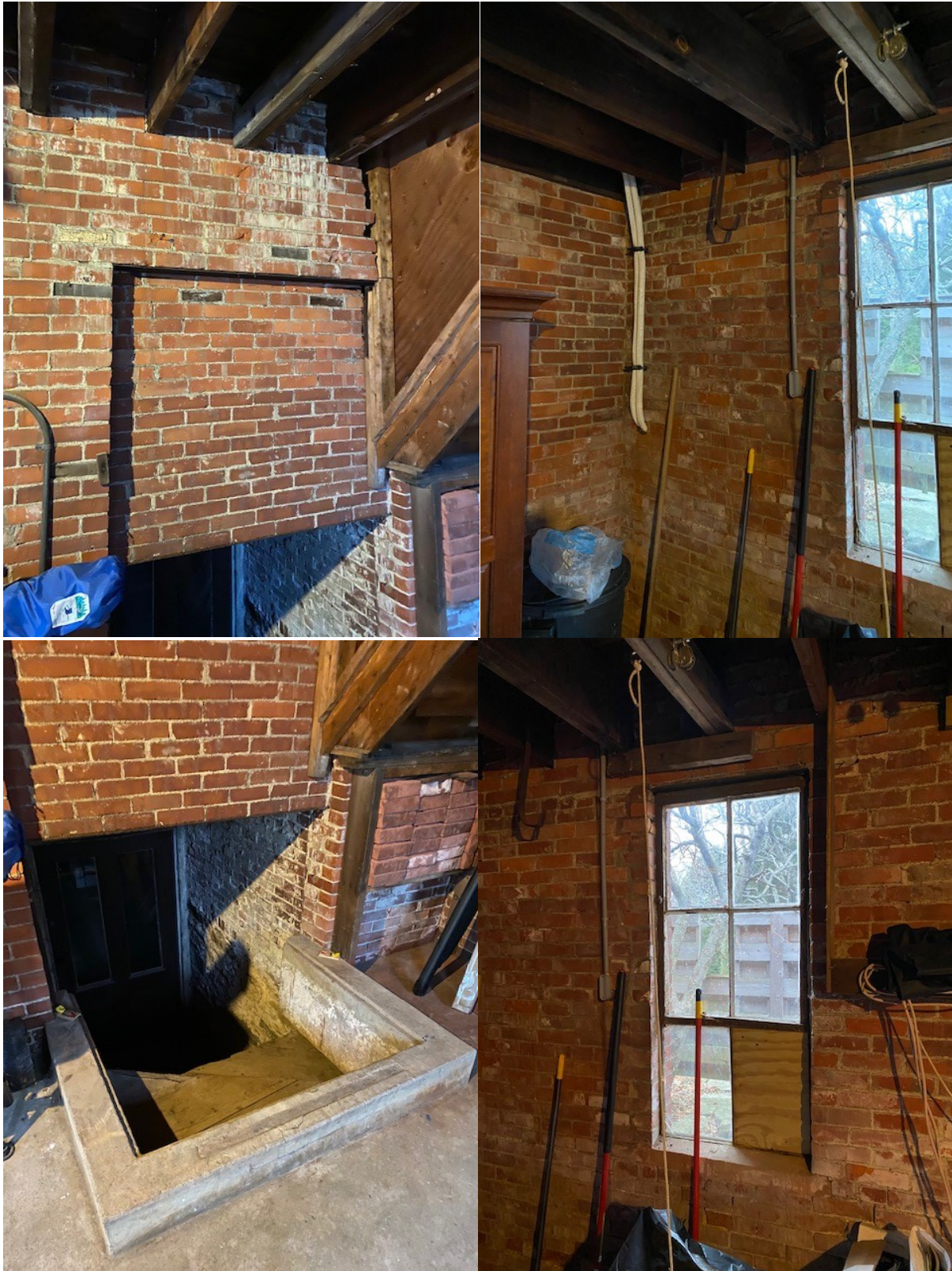
Interior brick in poor condition with some spalling. Concrete stair to the basement has winders, low headroom and irregular riser sizes. Dangerous access point.
