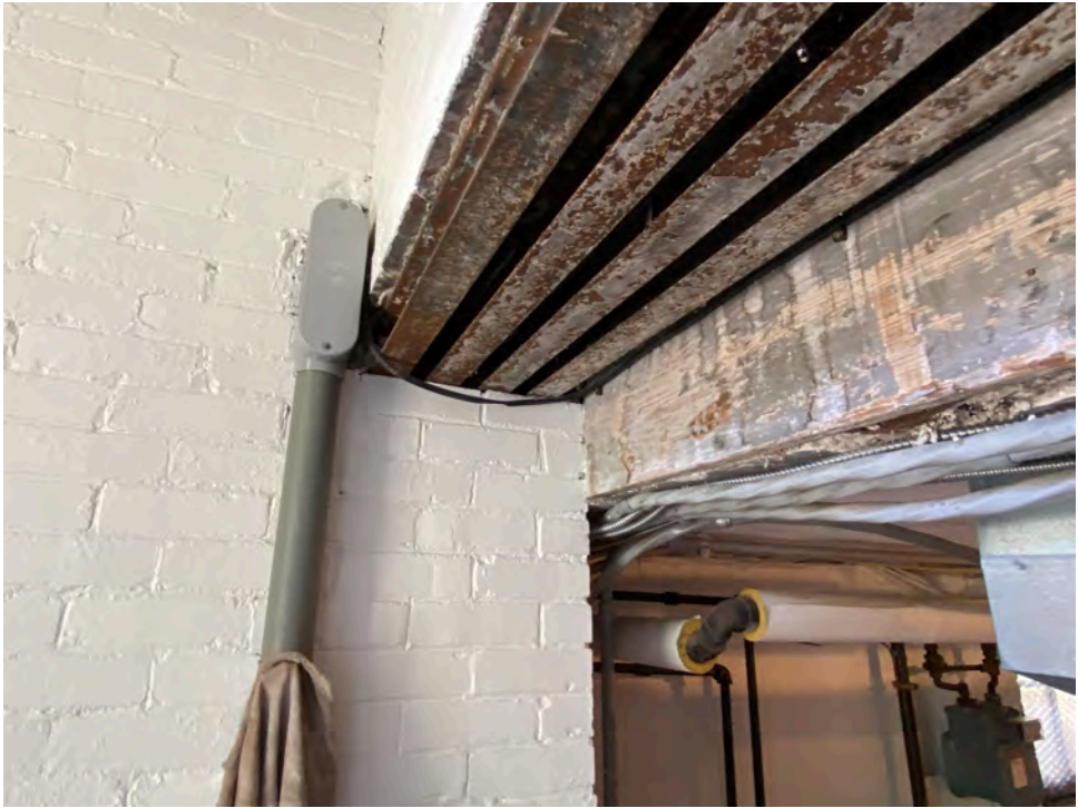
Obstructions: steel beams, wood floor joists, ductwork
