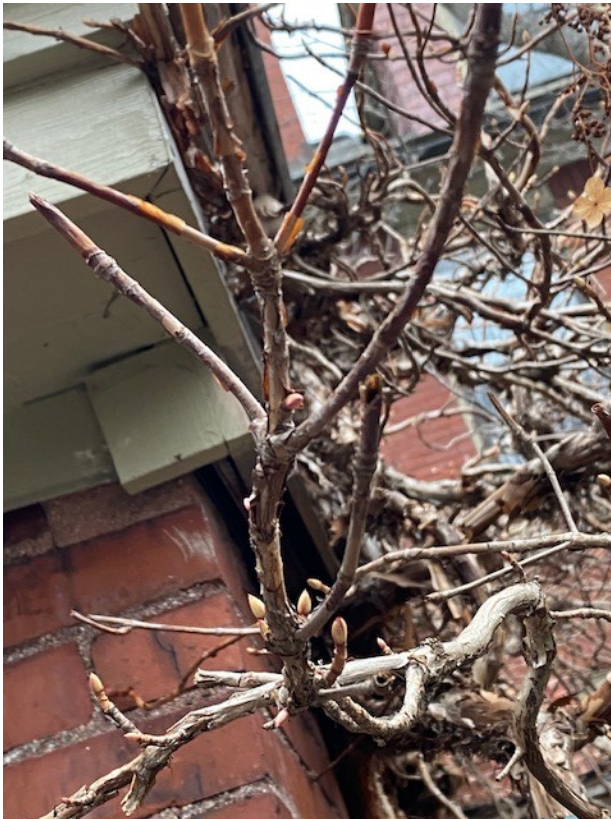
Duplex neighbors climbing Hydrangea on the East side is causing damage to the brickwork.
