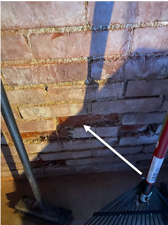
Picture #1: Spalling Brick
