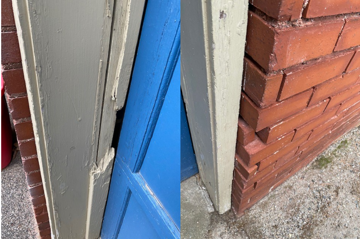
Exterior trim, jamb at the garage door has broken components. Brick work is missing mortar and brick.
