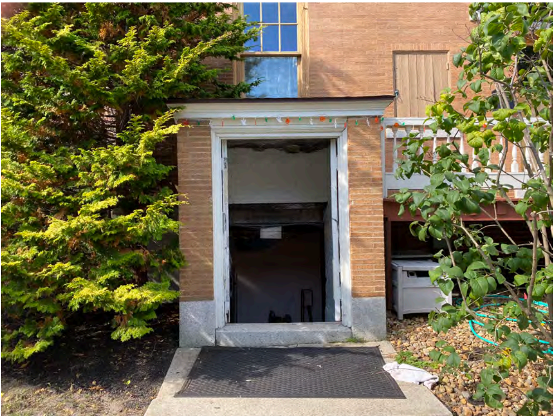
Open doors show obstructions that limit access for large items
