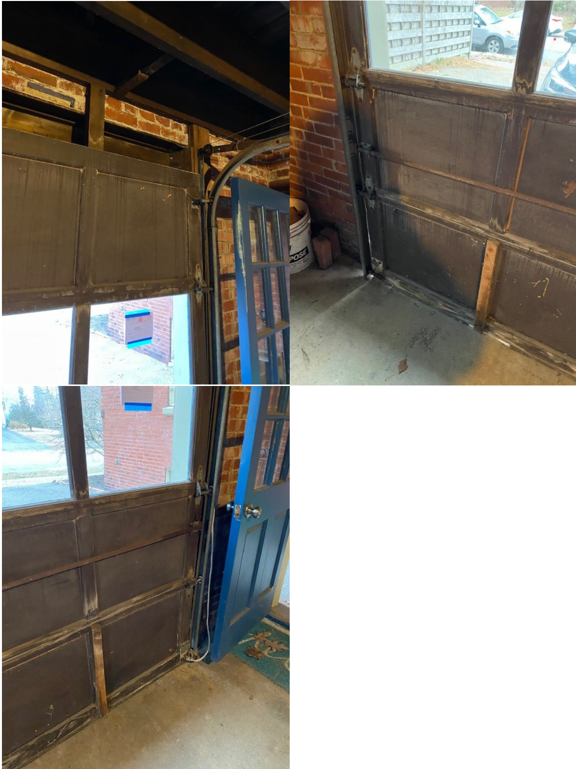
Wood garage door in poor condition.
