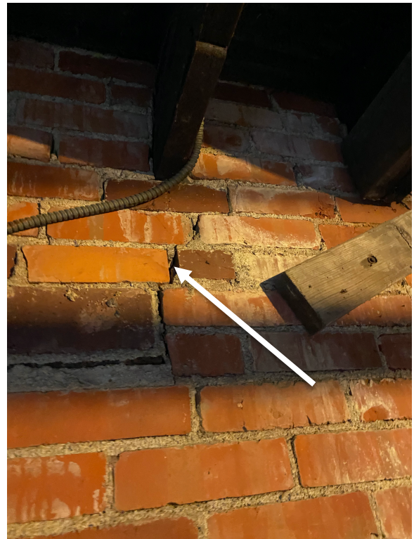
Picture #2: Large Brick Crack
