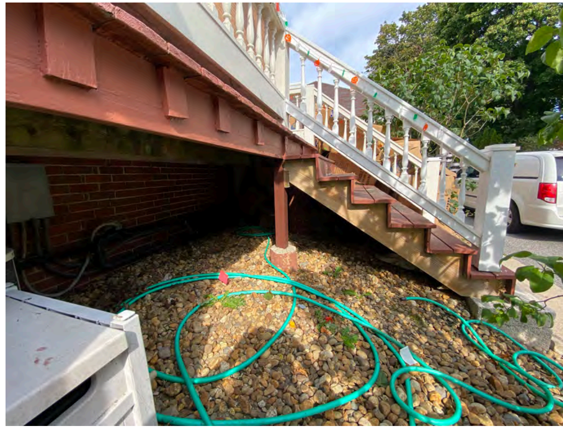
Poor construction of the existing porch and stair
