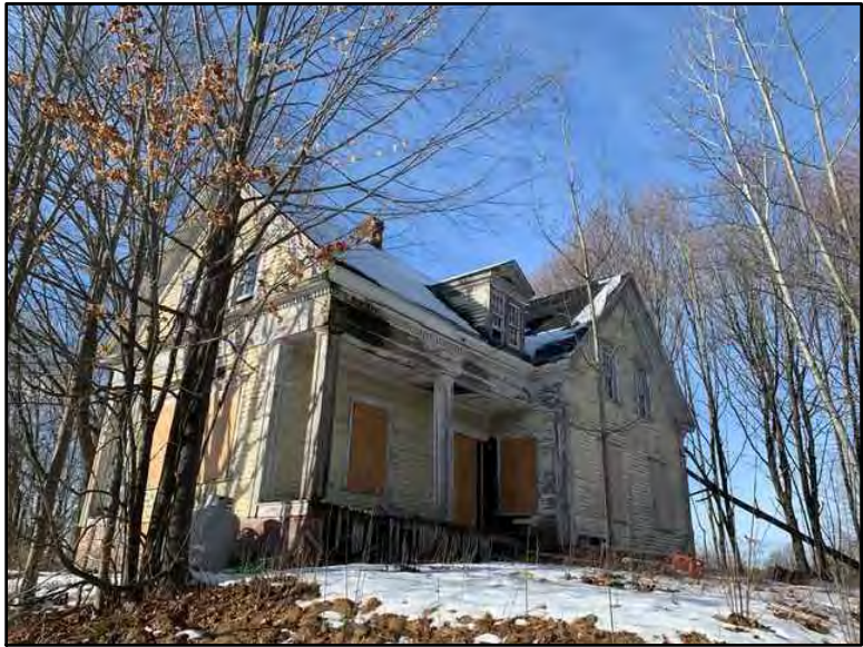
③ CONDITION OF HOME AT PURCHASE
