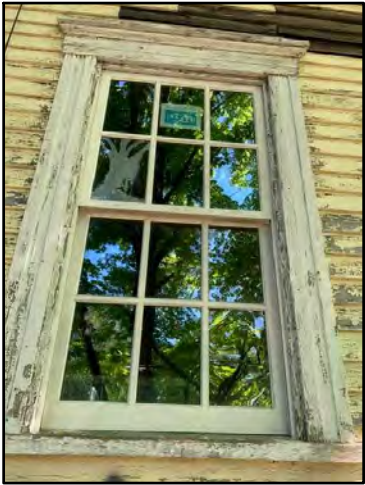
4 ORIGINAL EXTERIOR TRIM WITH PRIOR OWNER'S SASH INSERTED
