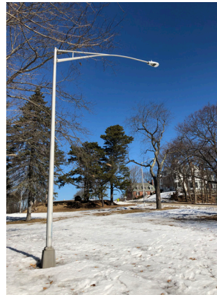
(top) Existing street lighting and walkway lighting
