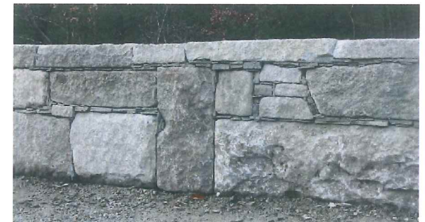
Random rectangular stones with consistent capstone. (This example has too many shims and is too tall)
