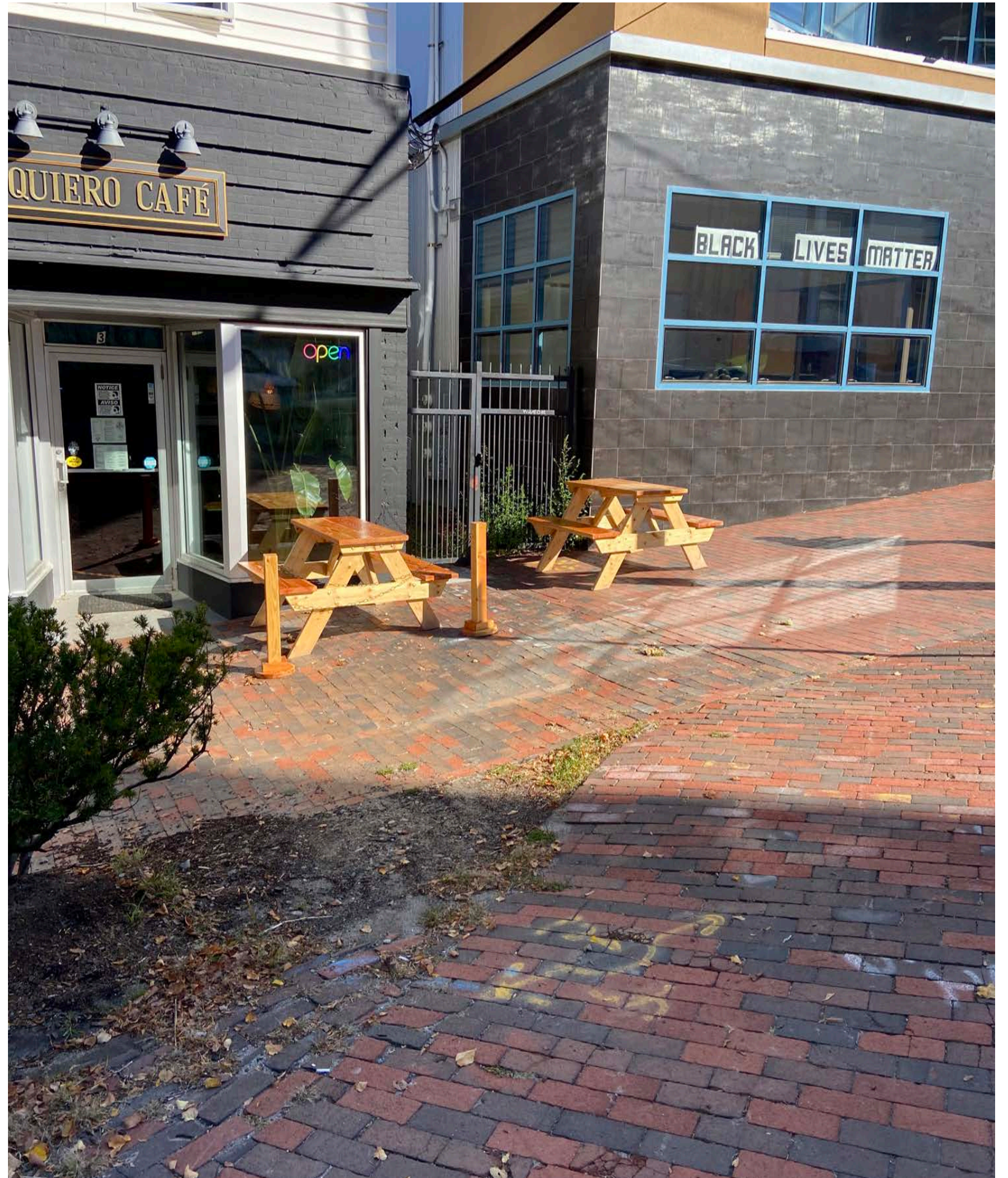
Accessibility and grading issues- existing condition does not provide a minimum 2% cross-slope
