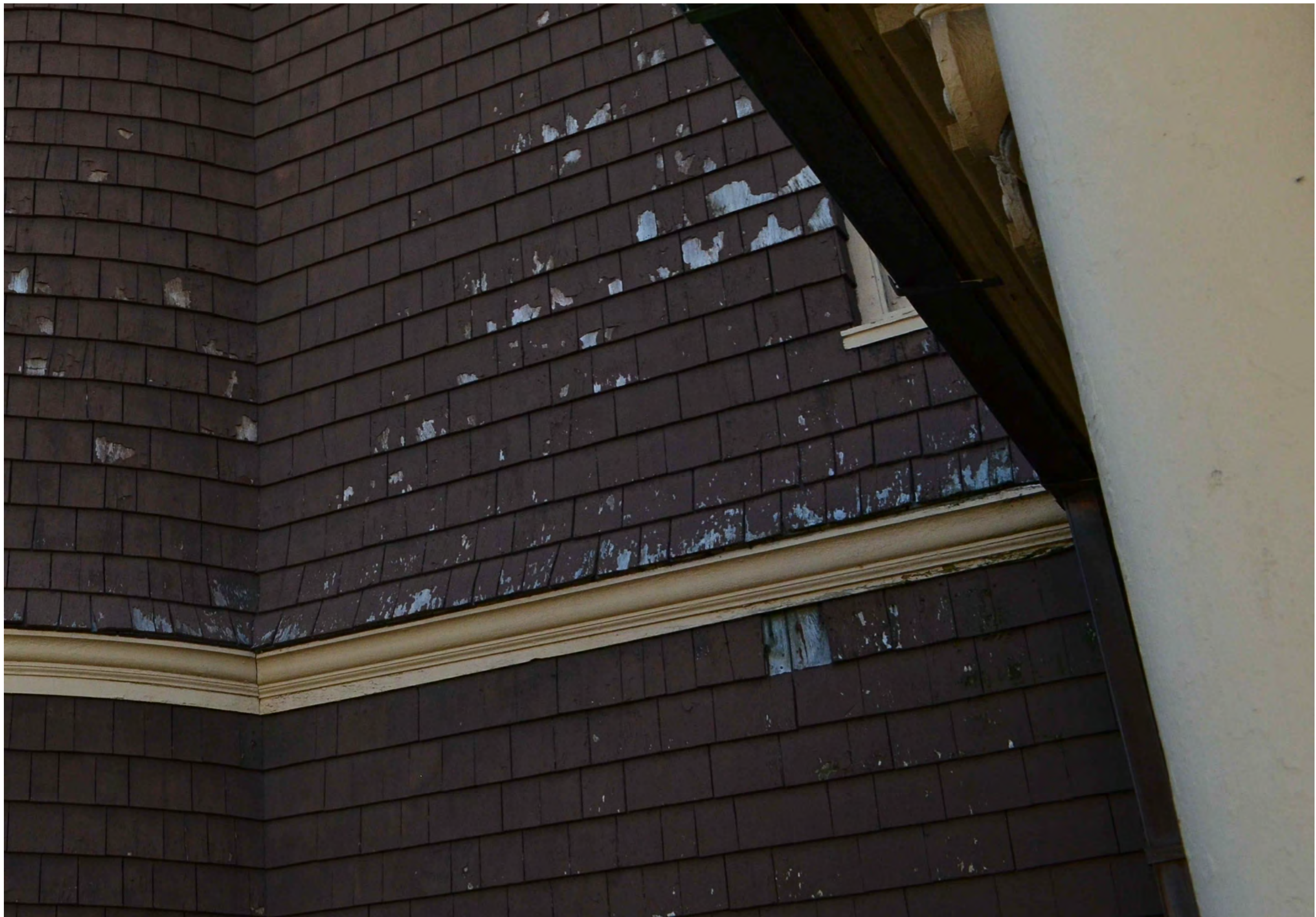
J. MISSING SHINGLE TO BE REPLACED ON LEFT SIDE OF PORCH, FROM NORTH ELEVATION.
