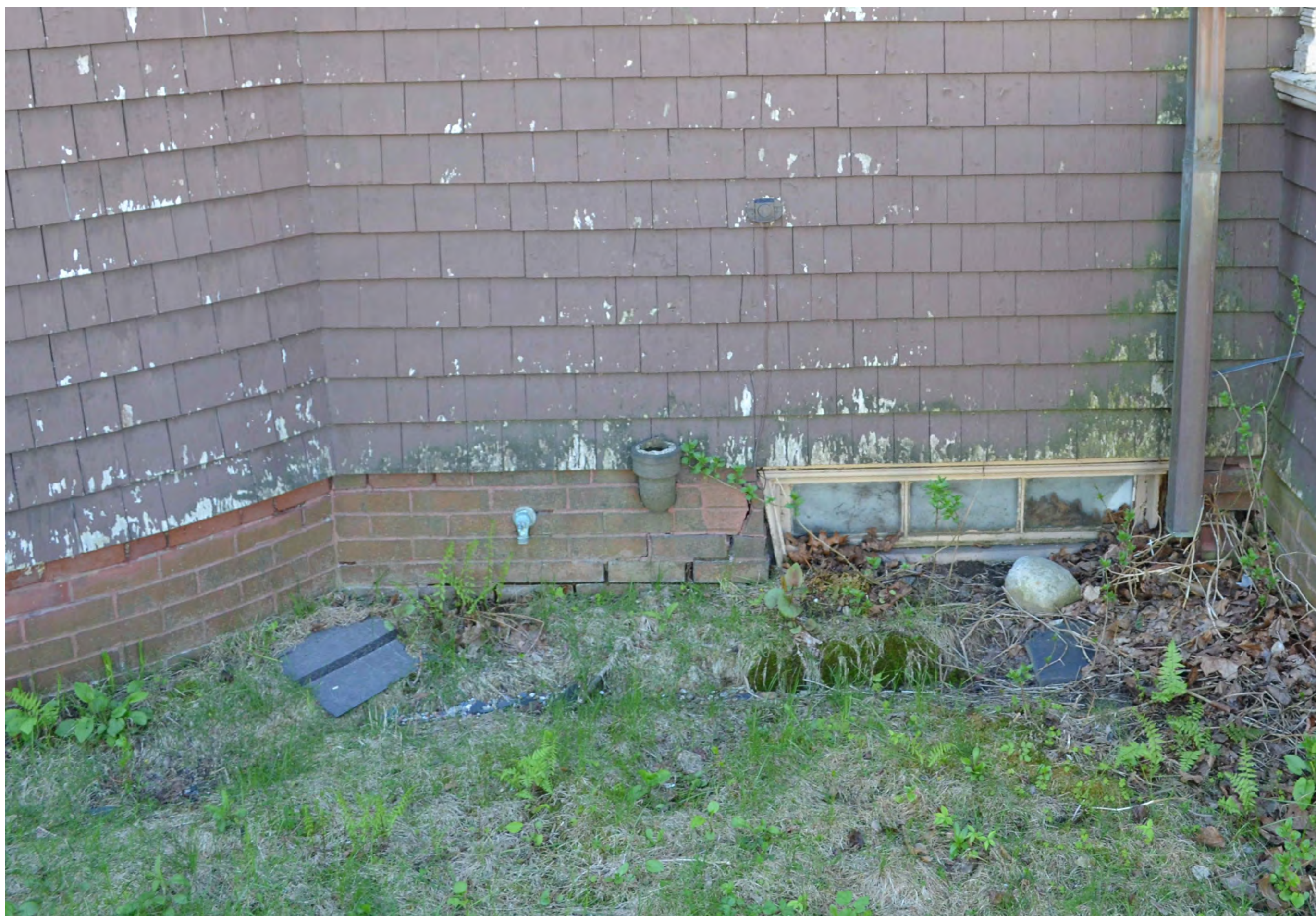
C. DETERIORATED BRICK FOUNDATION, FROM NORTH ELEVATION.
