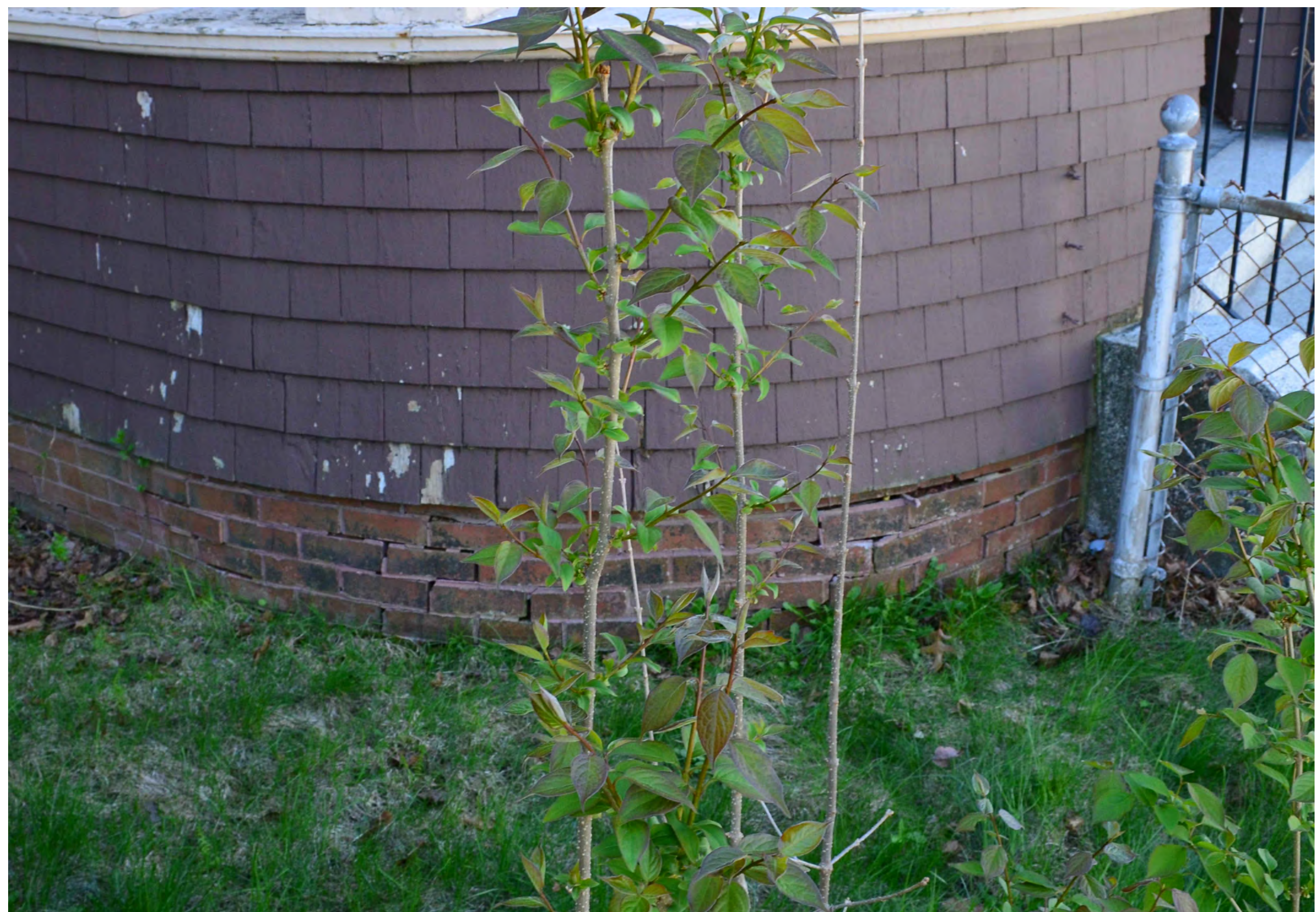
D. DETERIORATED BRICK FOUNDATION ON LEFT SIDE OF PORCH, FROM NORTH ELEVATION.
