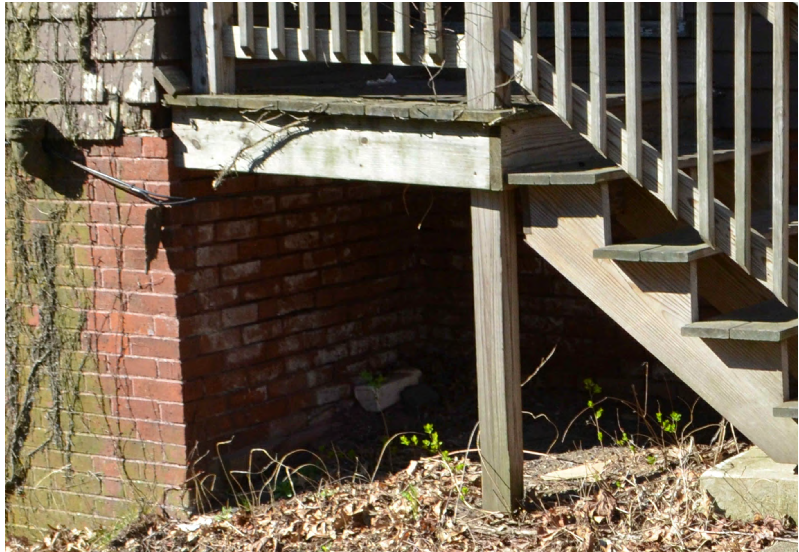
B. SALT DAMAGED BRICK UNDER SIDE ENTRANCE, FROM EAST ELEVATION.
