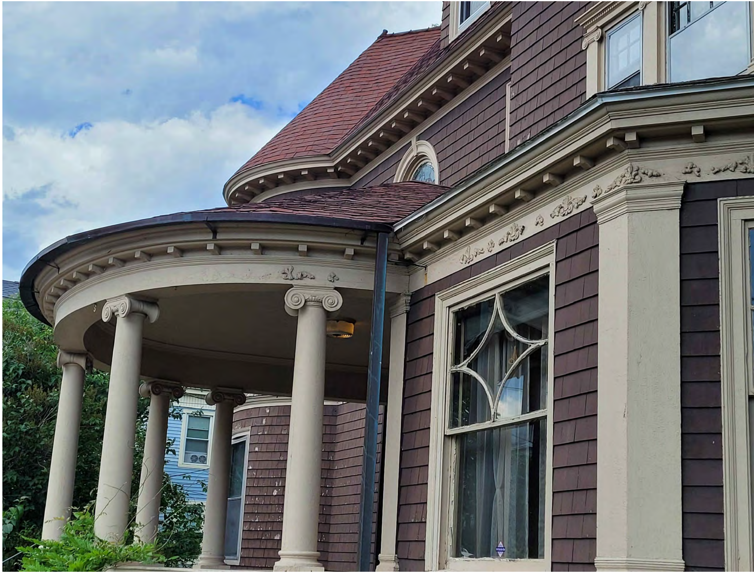
L. MISSING SCROLLING ON FASCIA, FROM NORTH ELEVATION.
