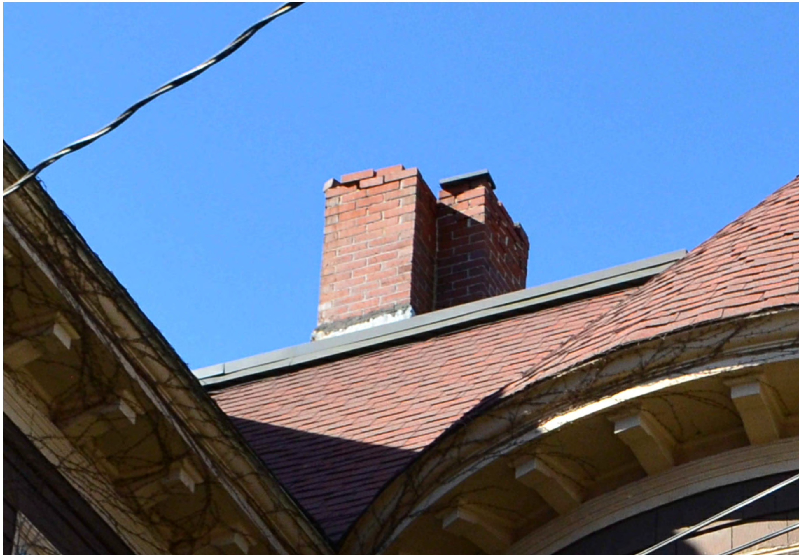
A. DETERIORATED BRICK CHIMNEY, FROM NORTHEAST ELEVATION.
