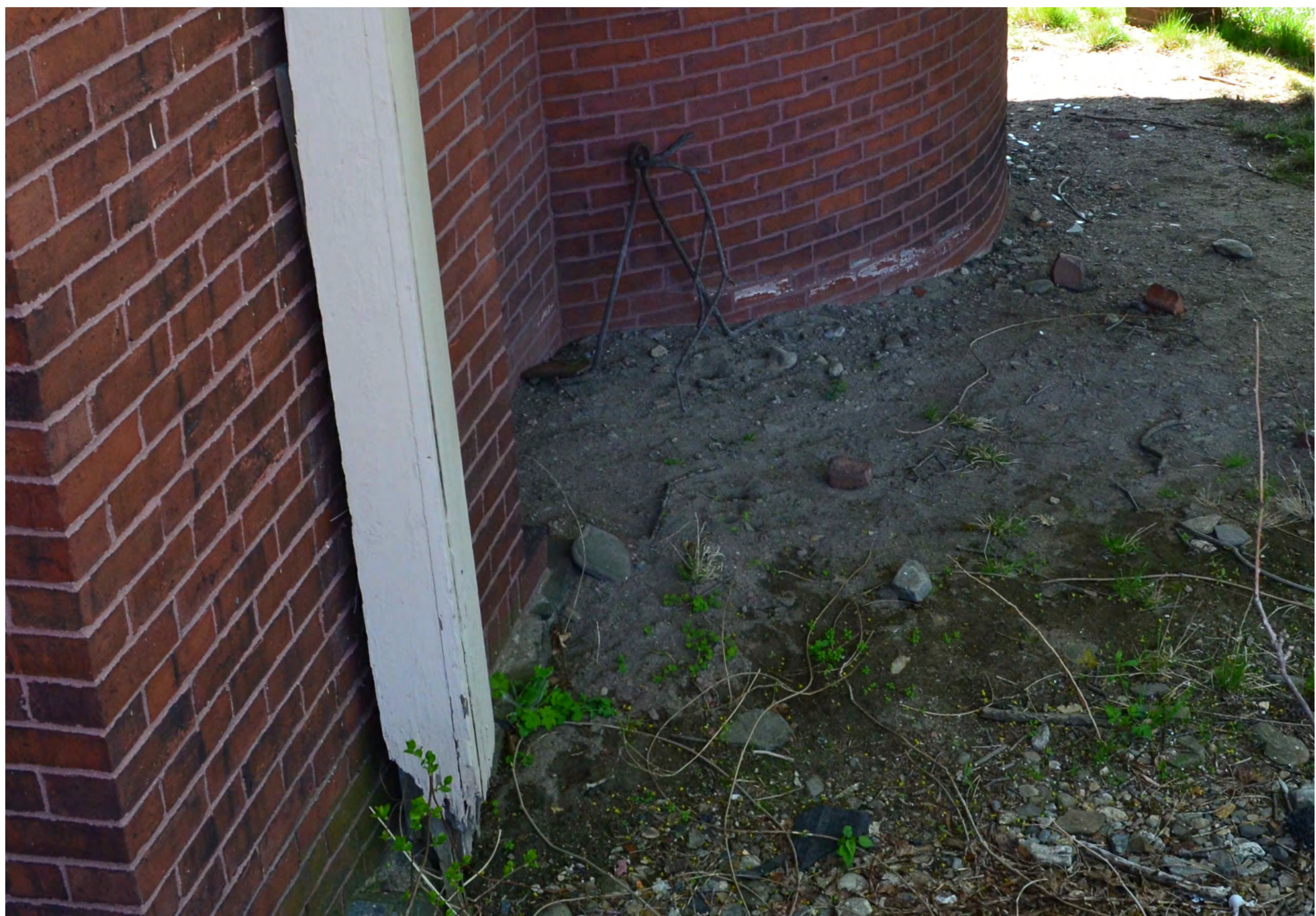
CC. WOOD POST TO BE REPLACED, FROM WEST ELEVATION.
