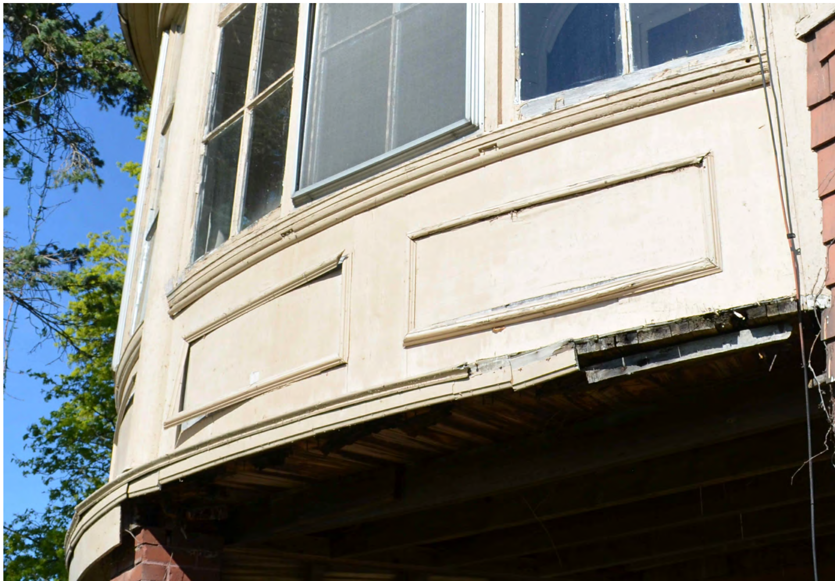
Q. DAMAGED TRIM TO BE REMOVED AND REPLICATED, FROM SOUTH ELEVATION.
