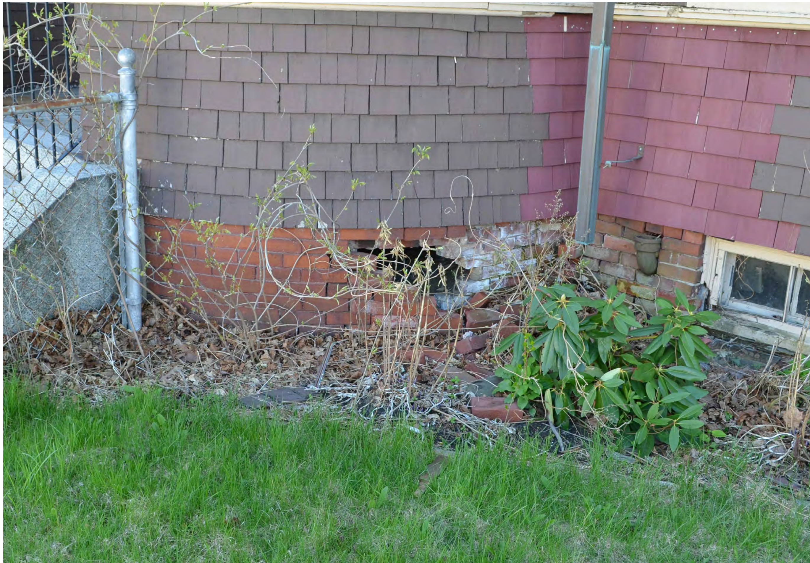
E. DETERIORATED BRICK FOUNDATION ON RIGHT SIDE OF PORCH, FROM NORTH ELEVATION.
