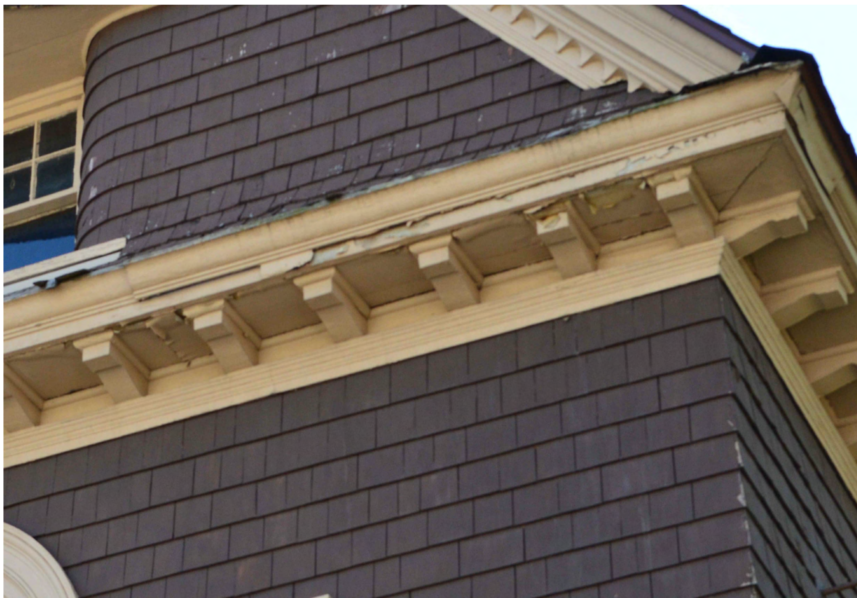
G. DETERIORATED WOOD CROWN MOLD TO BE REPLICATED, FROM NORTH ELEVATION.
