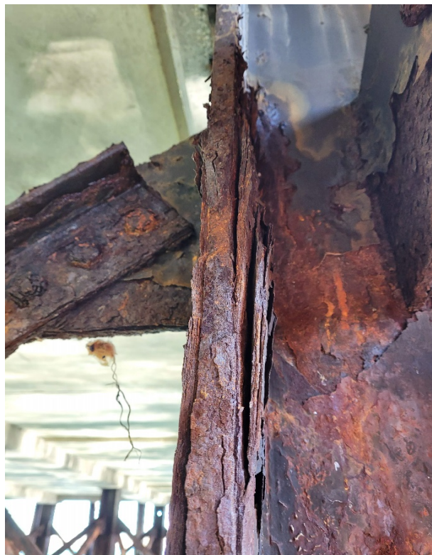
Picture #20 Typical heavy scale and corrosion at sorting piers
