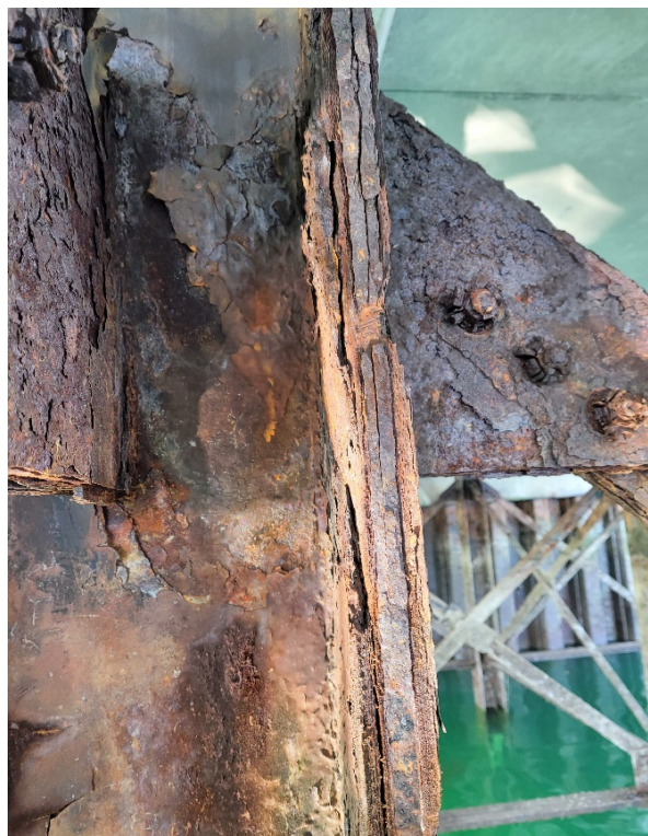
Picture #24 Heavy scale and corrosion at Sorting Pier 3
