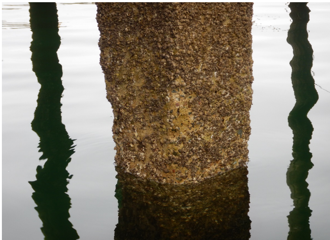
Picture #30 Concrete pile section loss
