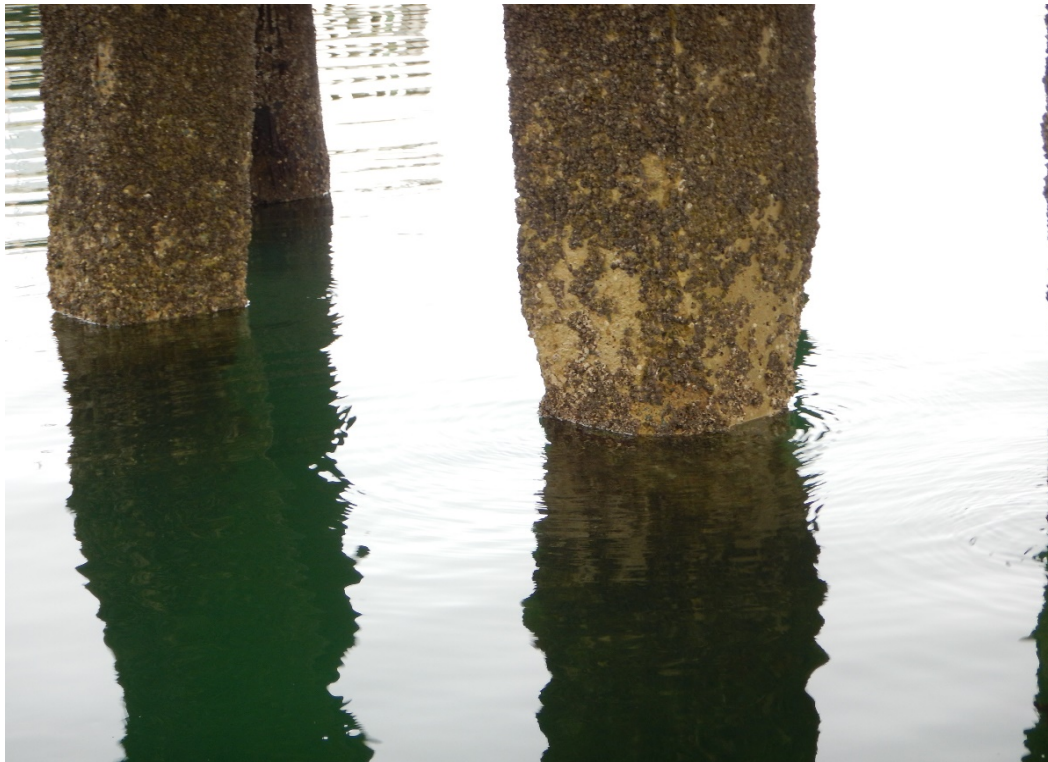
Picture #29 Concrete pile section loss
