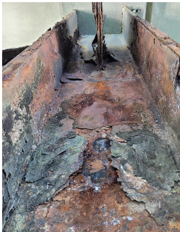
Picture #22 Heavy scale and corrosion loss
