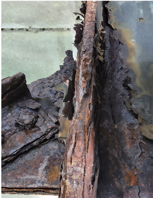
Picture #21 Heavy corrosion loss to H-pile flange
