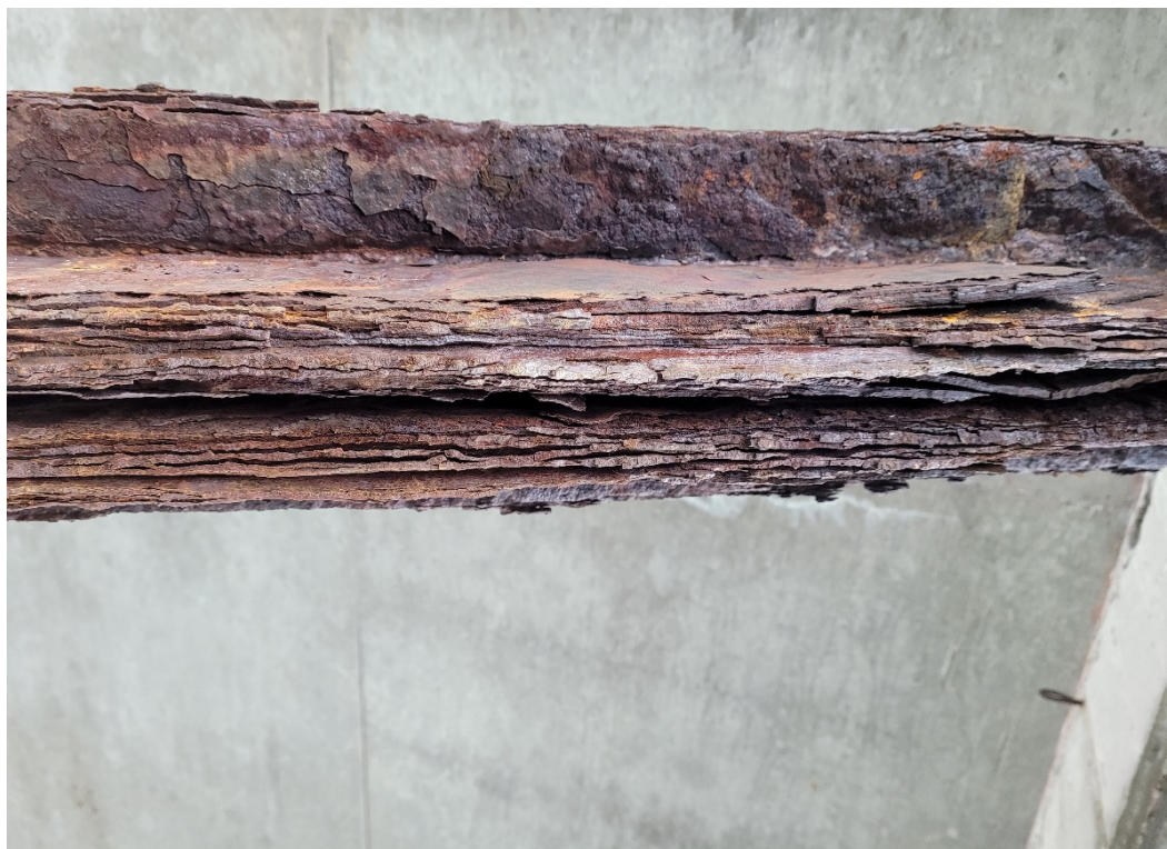
Picture #18 Typical heavy corrosion and scale to lateral diagonal bracing
