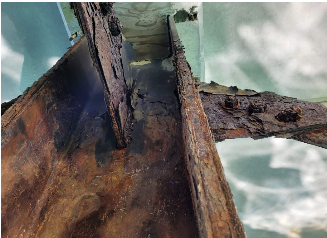
Picture #16 Typical conditions (poor)
