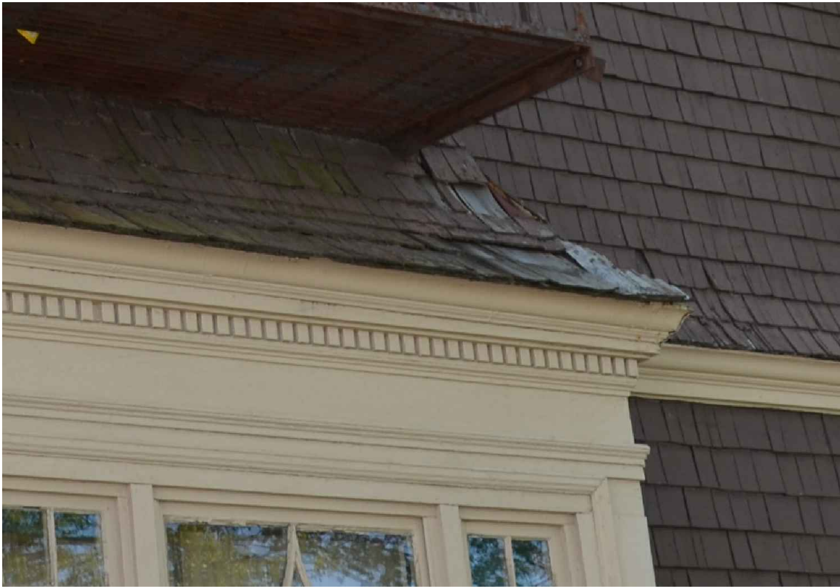
AA. SHINGLES TO BE REMOVED AND REPLACED ON BAY ROOF, FROM WEST ELEVATION.
