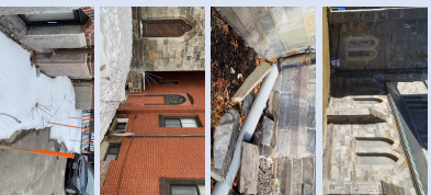
Existing Stormwater Run-Off Issues
