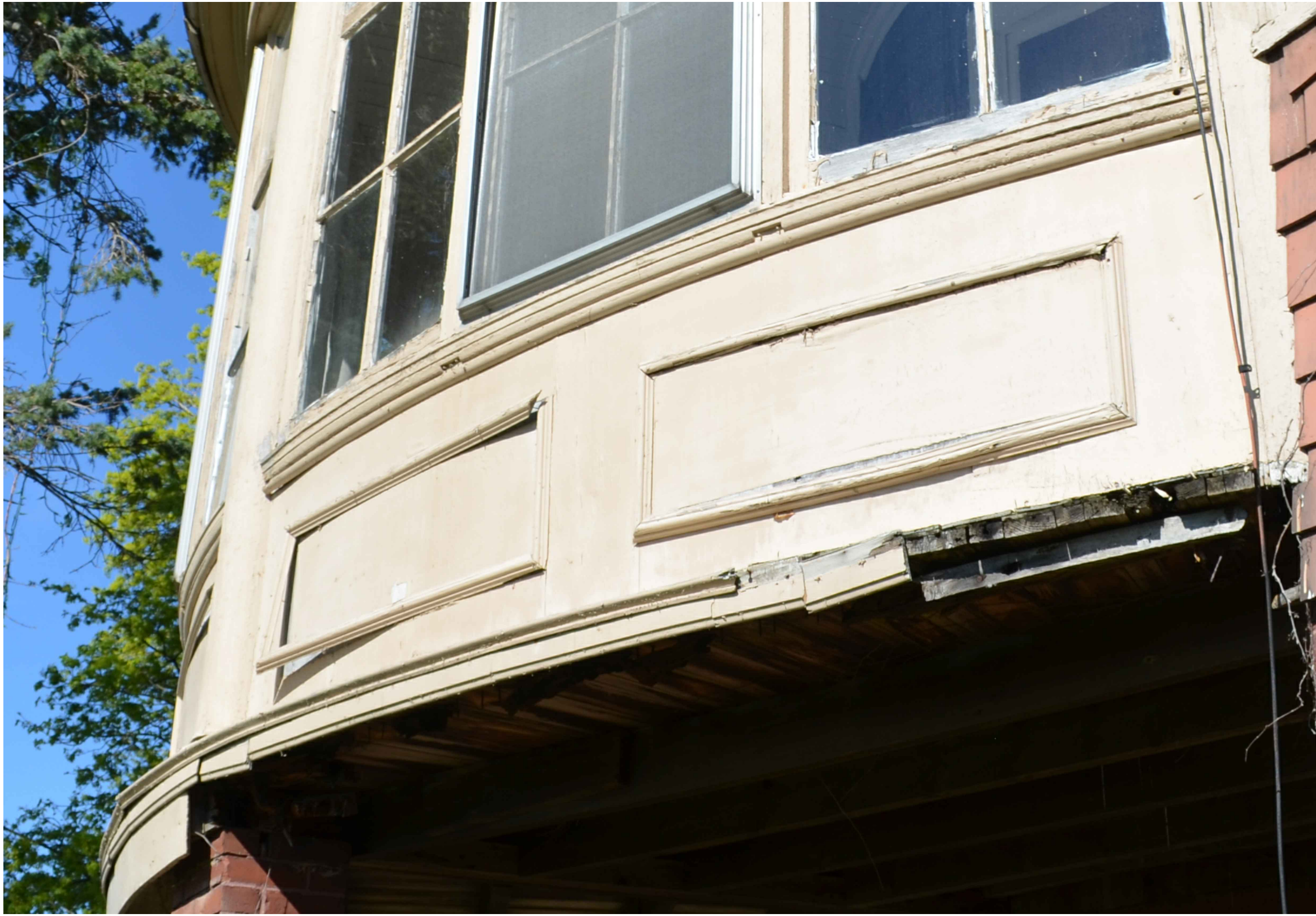
Q. DAMAGED PANELS TO BE REMOVED AND REPLACED (WITH BALLUSTERS), FROM SOUTH ELEVATION.
