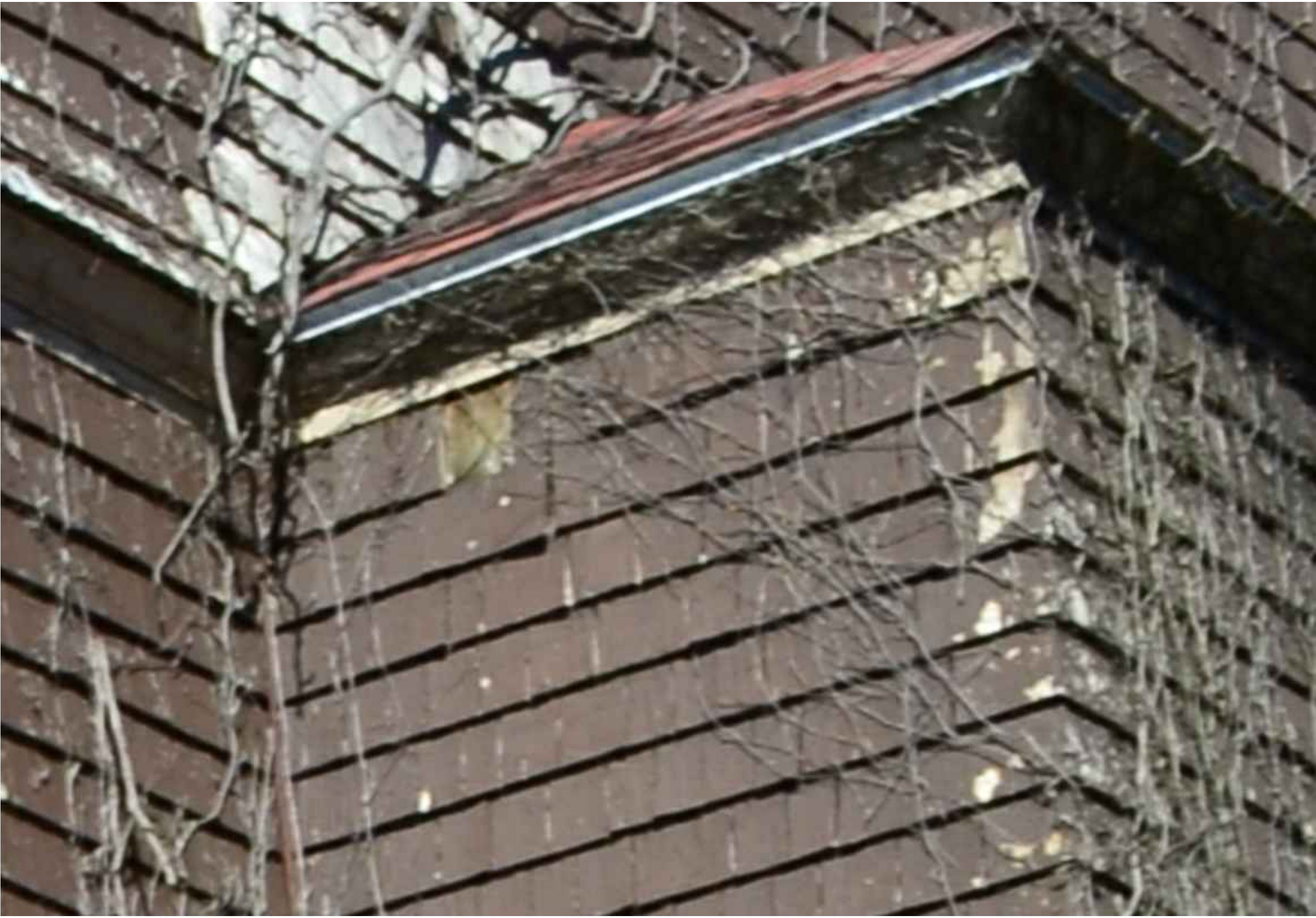
R. MISSING SHINGLE TO BE REPLACED, FROM SOUTH ELEVATION.
