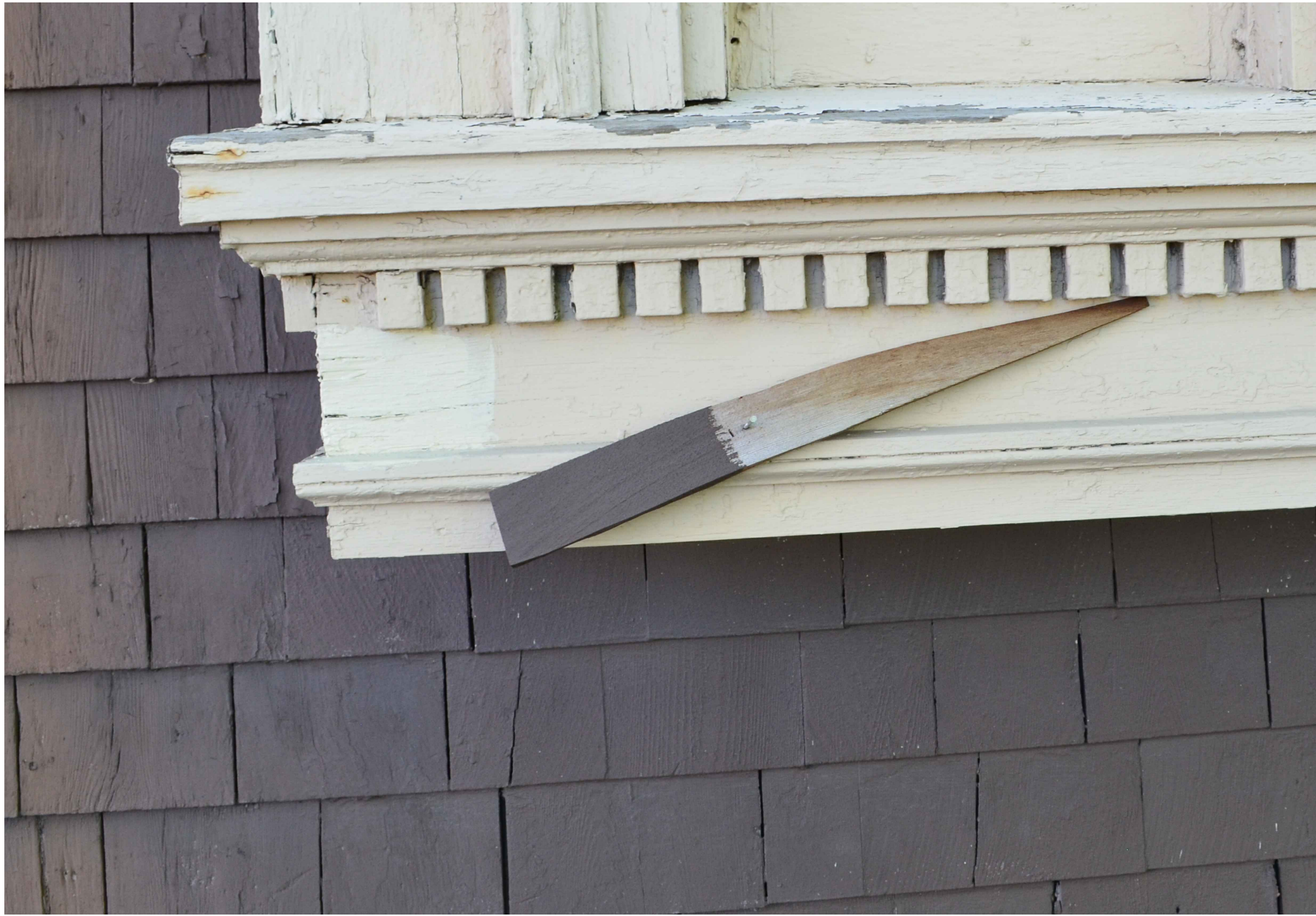
BB. WOOD TO BE REMOVED AND WOOD CROWN TO BE REPAIRED, FROM WEST ELEVATION.
