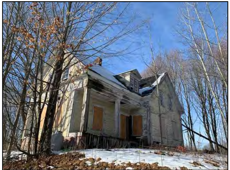
③ CONDITION OF HOME AT PURCHASE
