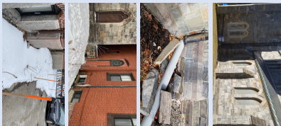
Existing Stormwater Run-Off Issues
