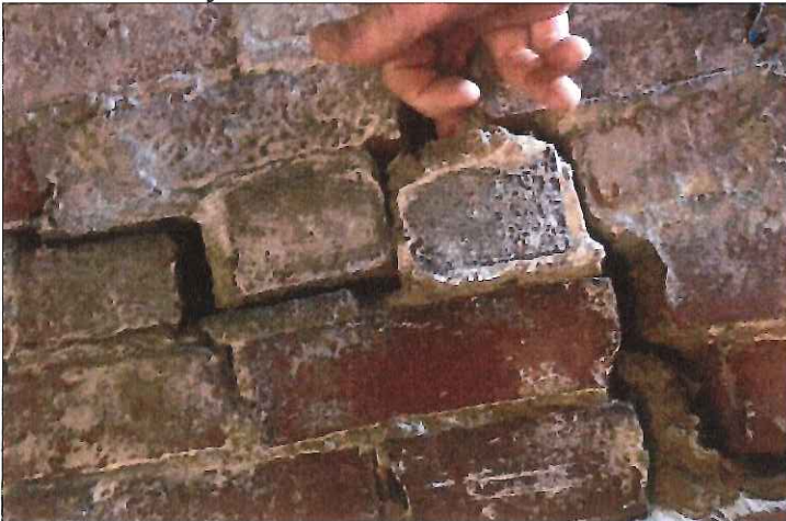
Existing Masonry Crack and sand from within masonry core
