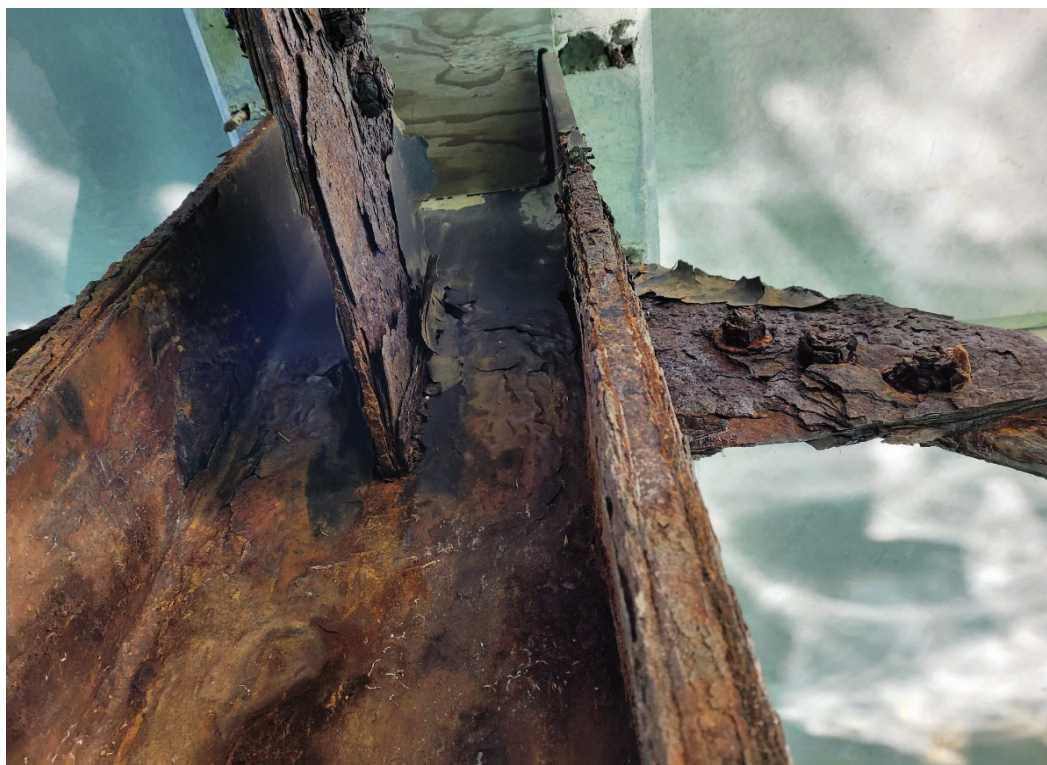
Picture #16 Typical conditions (poor)
