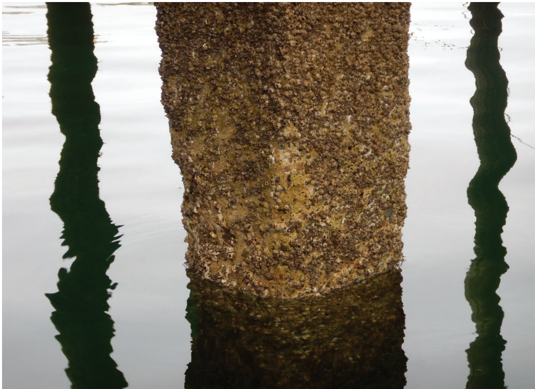
Picture #30 Concrete pile section loss
