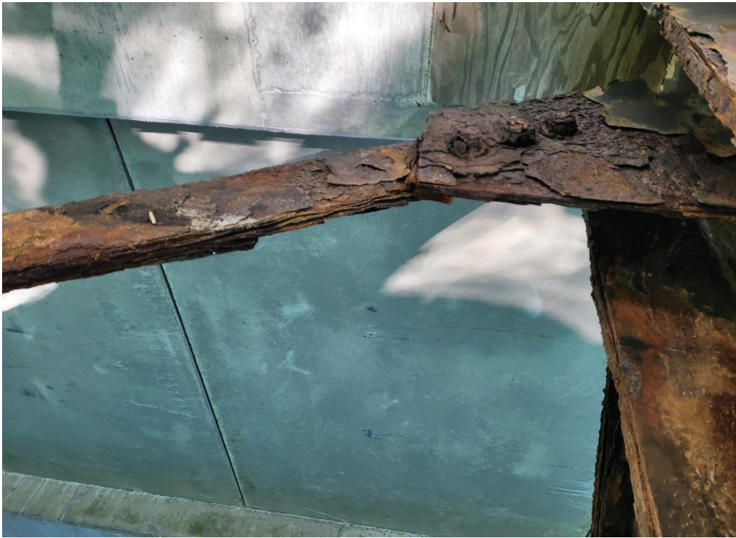
Picture #17 Typical heavy corrosion and scale to longitudinal diagonal bracing
