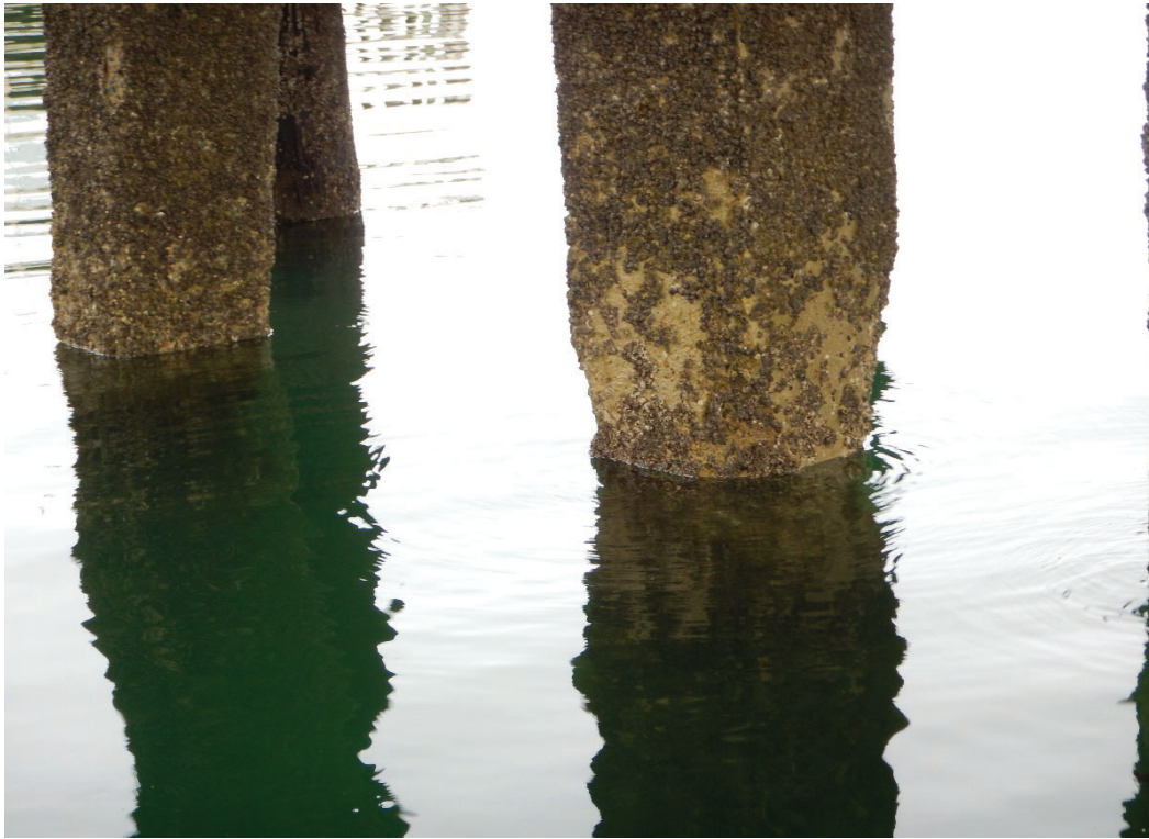
Picture #29 Concrete pile section loss
