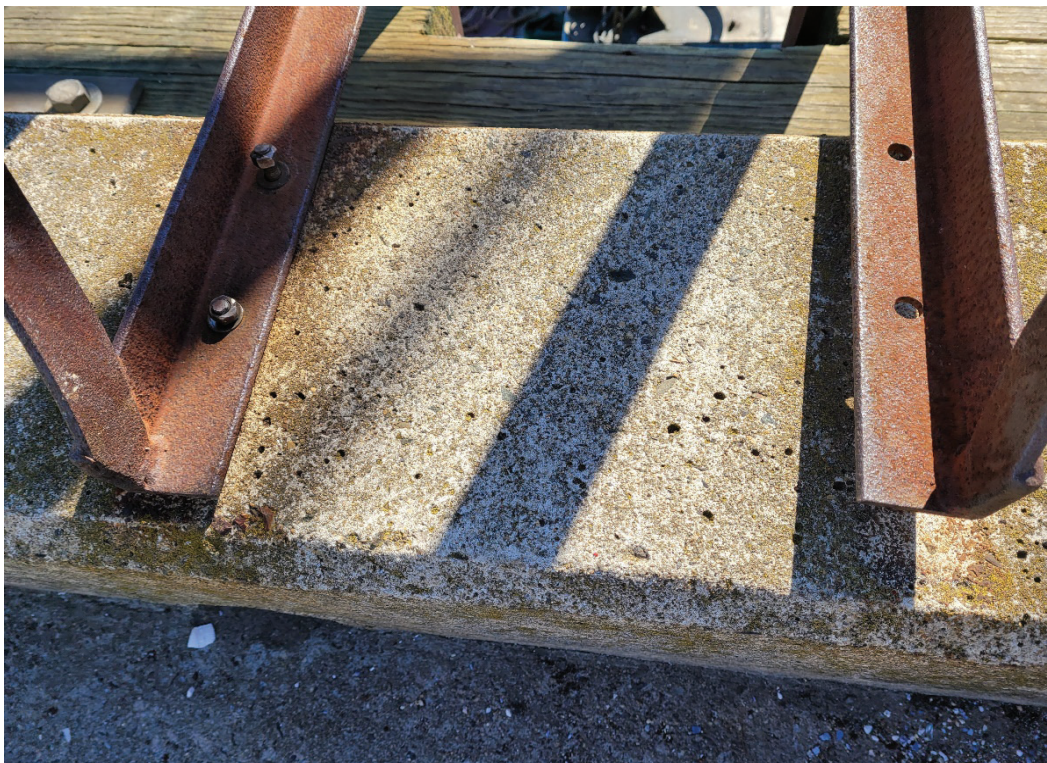
Picture #10 Loose/missing ladder bolts at Sorting Pier 3 Extension
