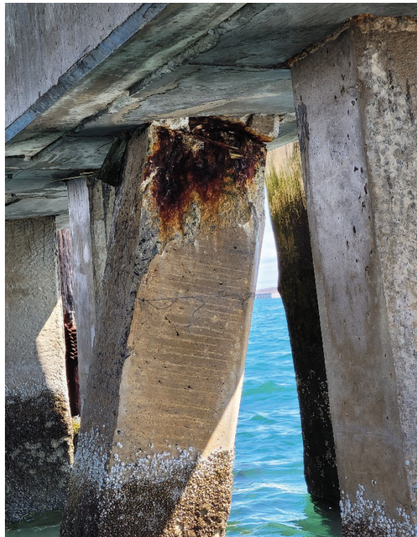
Picture #28 Sorting Pier 1 Extension, Bent 5, Pile 5
