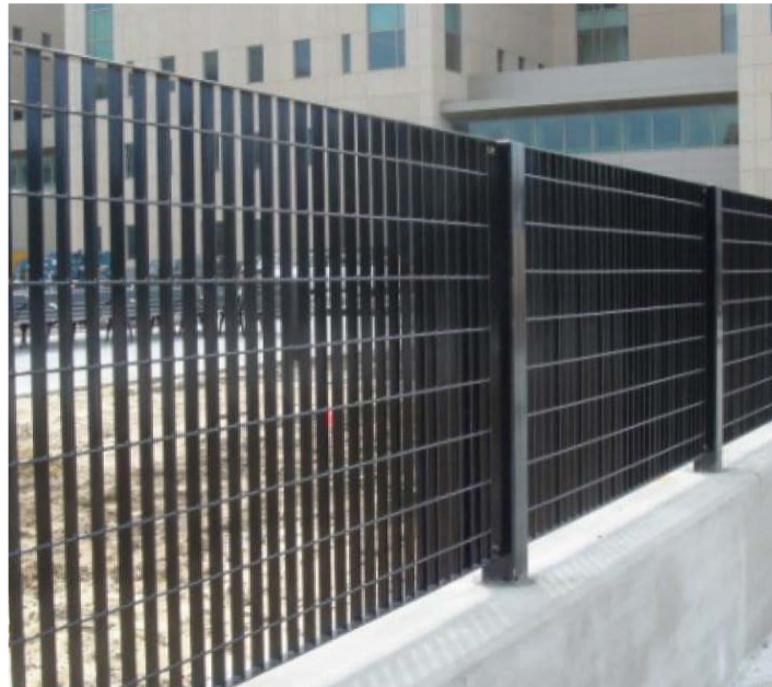
SECURITY GRILLES AND STAIR GUARDS
