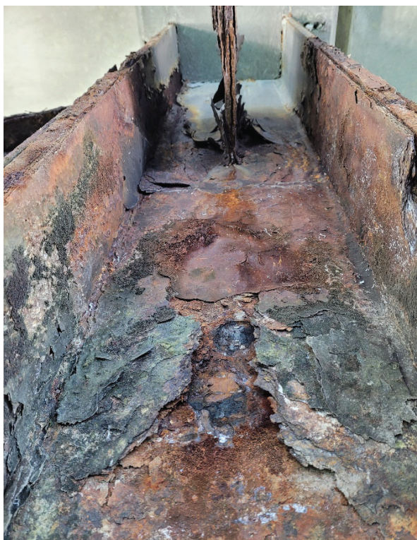
Picture #22 Heavy scale and corrosion loss
