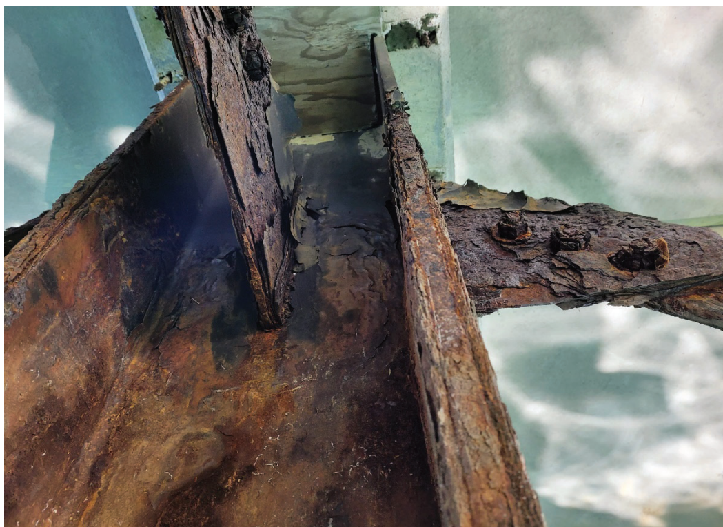
Picture #16 Typical conditions (poor)
