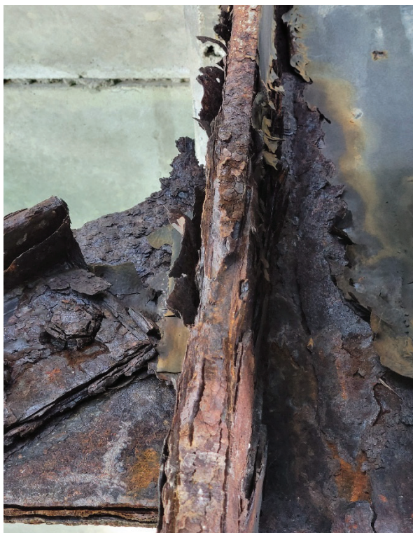
Picture #21 Heavy corrosion loss to H-pile flange
