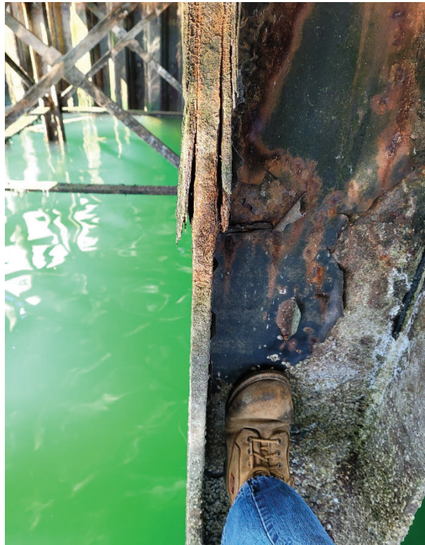
Picture #19 Typical scale and corrosion at sorting piers
