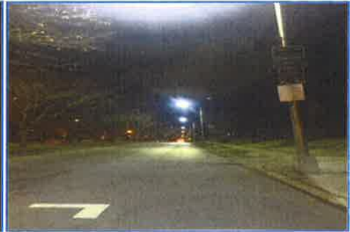
Baltimore After – LED Cobra Head Luminaires
