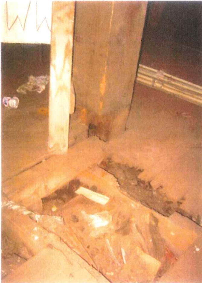
Photo 12-4: Rotting column bottom, floor joists and sills at ground floor.
