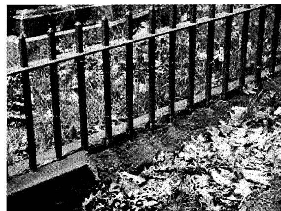
Rust jacking damage at family plot edging
