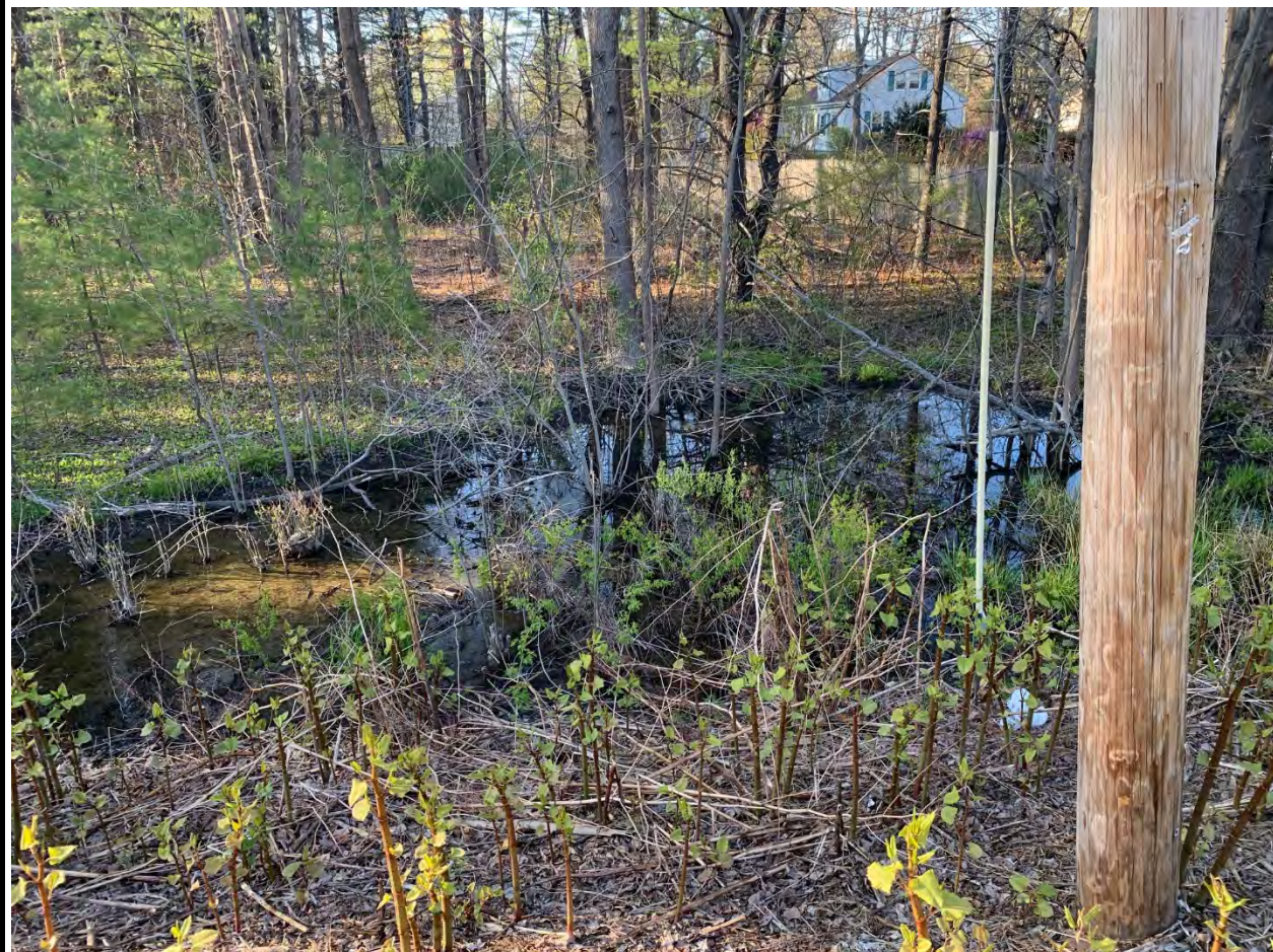
Drainage/Pooling Along Road – May 12, 2020
