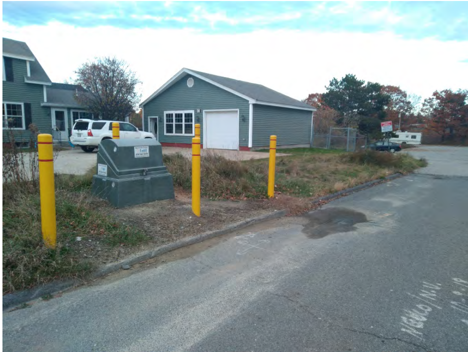
Figure 5. Until equipment at access driveway entrance, looking east.
