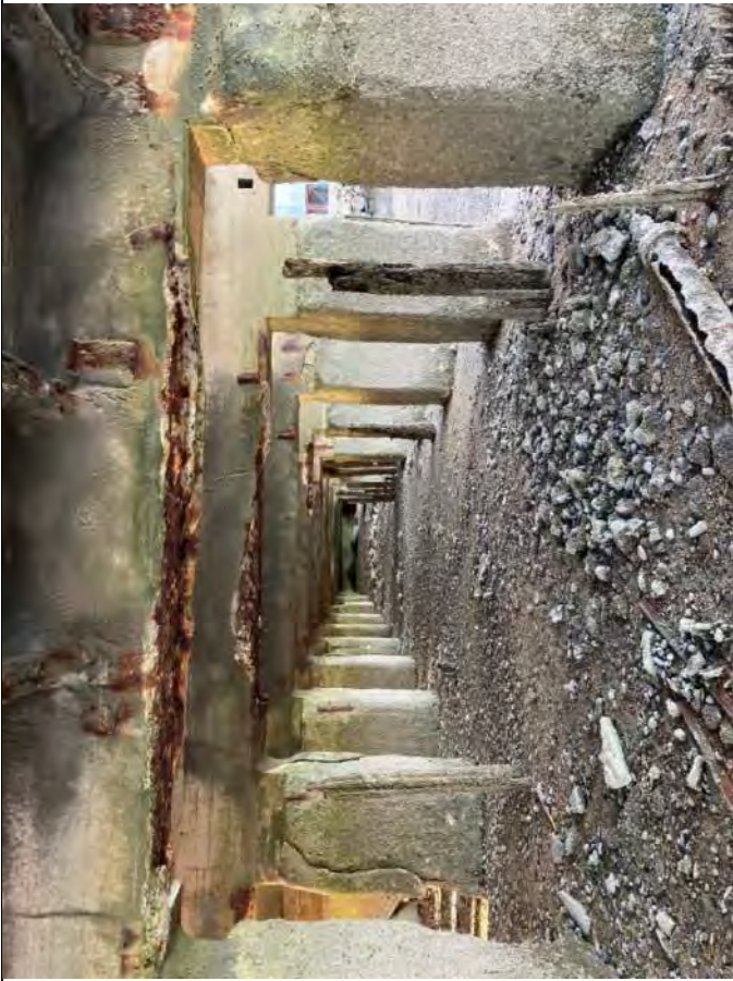
Photo 2 – First Floor Beam Corrosion Deterioration
