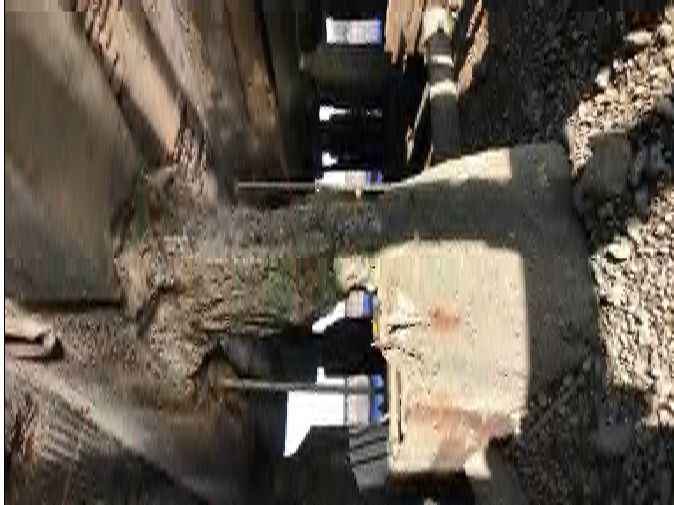
Photo 4 – First Floor Concrete Pier Deterioration
