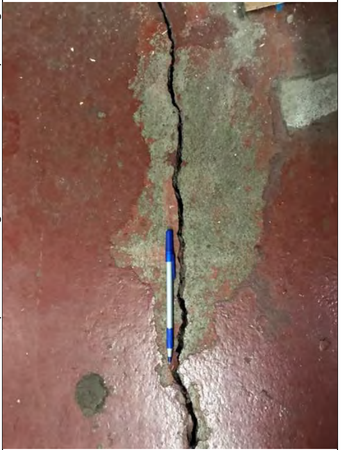
Photo 8 – Second Floor Slab Cracking
