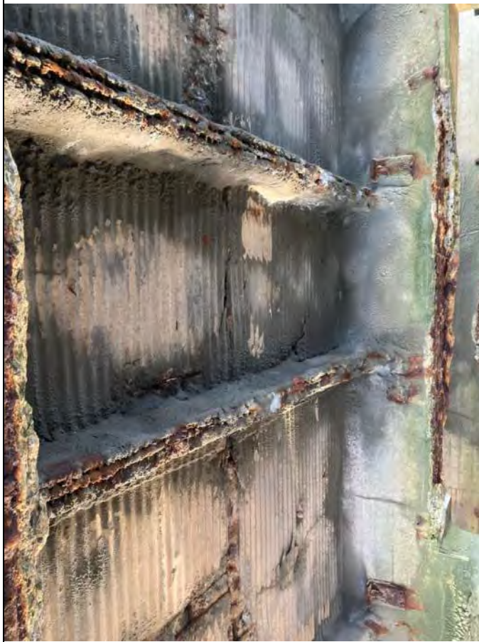
Photo 3 – First Floor Slab Corrosion Deterioration
