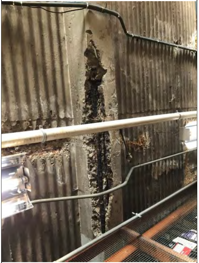
Photo 7 – Second Floor Slab and Beam Corrosion Deterioration
