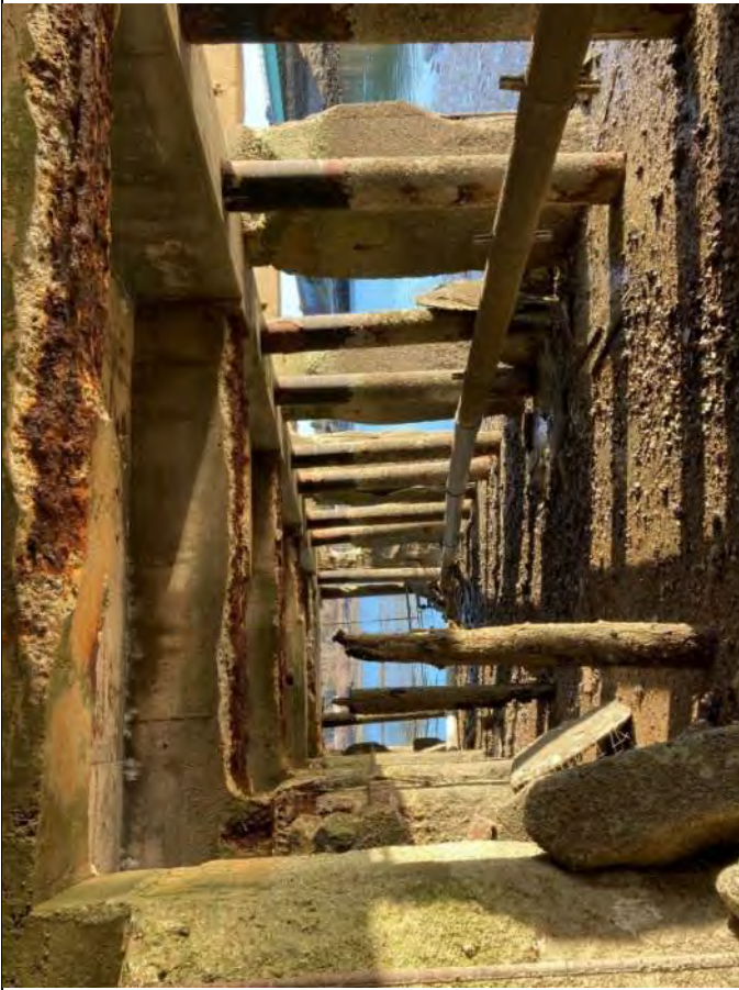
Photo 1 – First Floor Beam Corrosion Deterioration
