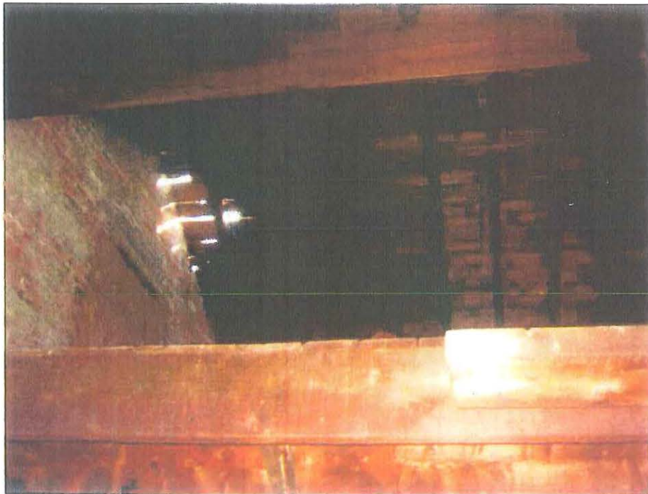
Photo 12-3: Daylight visible at through roof sheathing. Condition is at both ends of roof.
