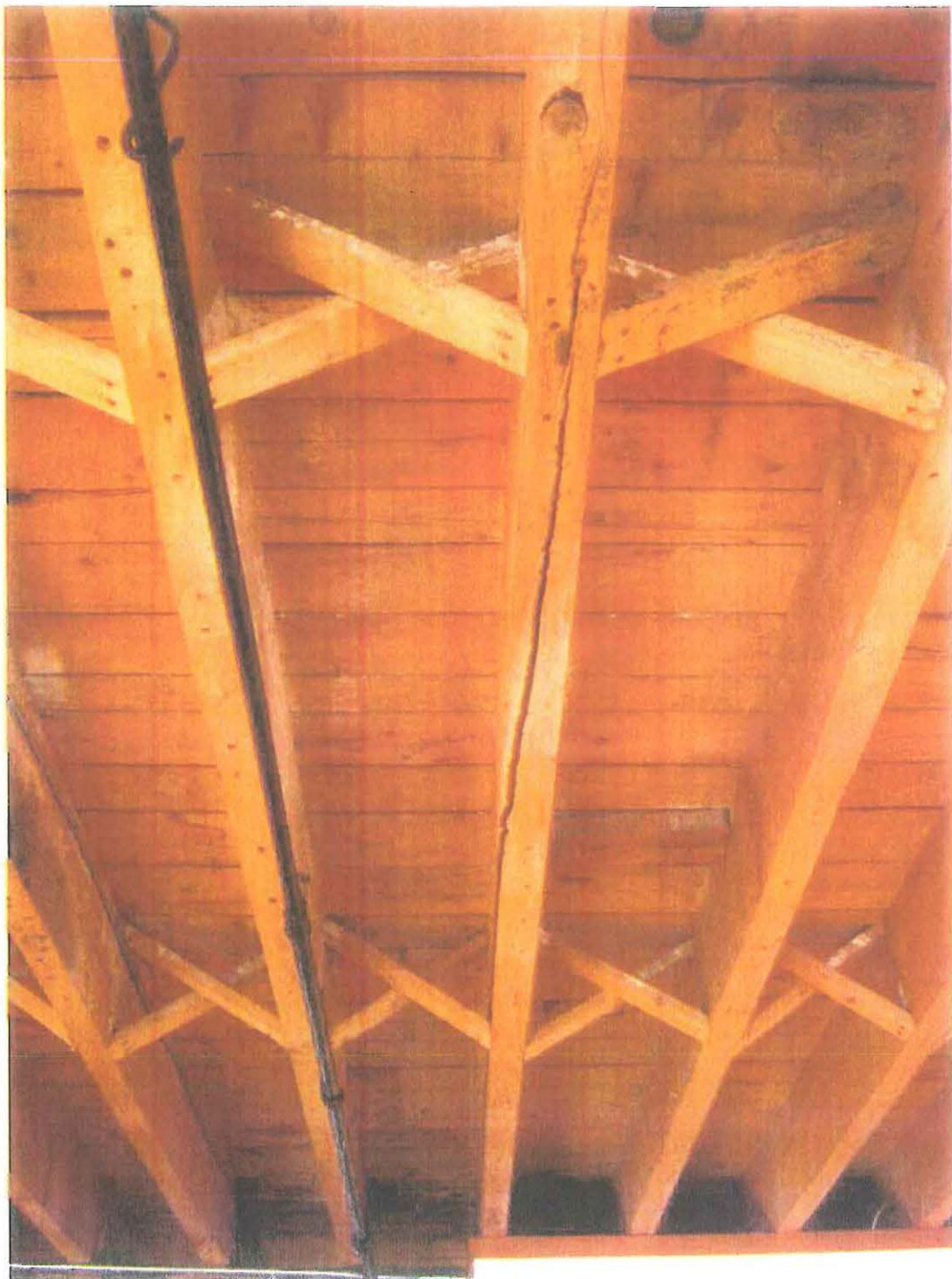
Photo 6A-4: Floor joist splitting.
