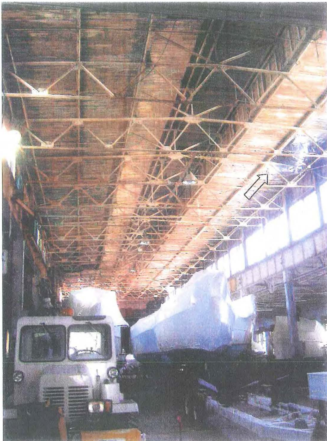
Photo 4-3: View of Building 4 interior looking east. Note plastic leak catch.
