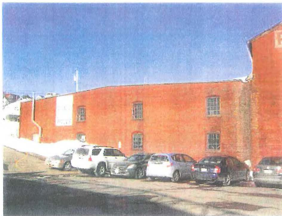
Photo 11-2: West elevation of Building 11. Note drainage condition where building 11 meets building 12.
