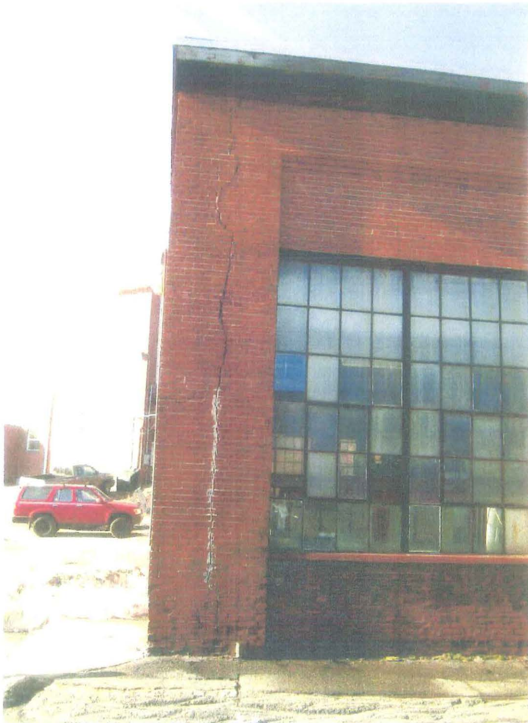
Photo 1-4: Vertical brick masonry crack at southwest pilaster.
