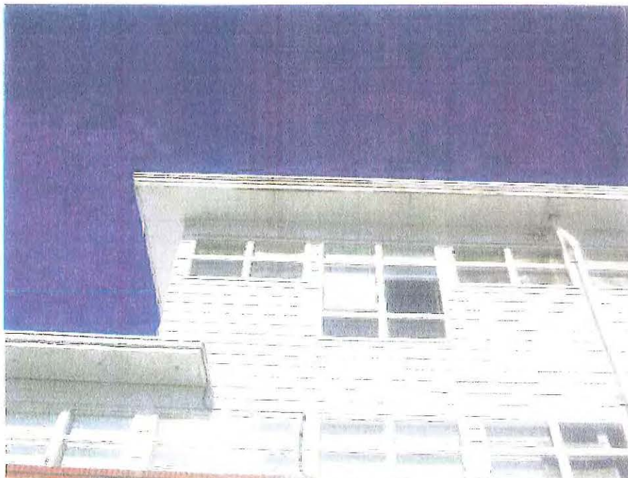
Photo 30-2: Peeling paint at roof eave, uneven siding.
