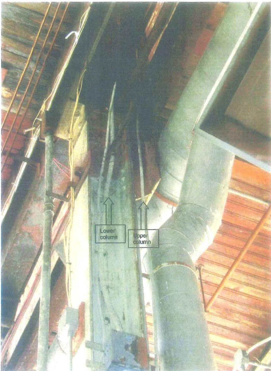
Photo 1-5: Column discontinuity at low-high roof condition.
