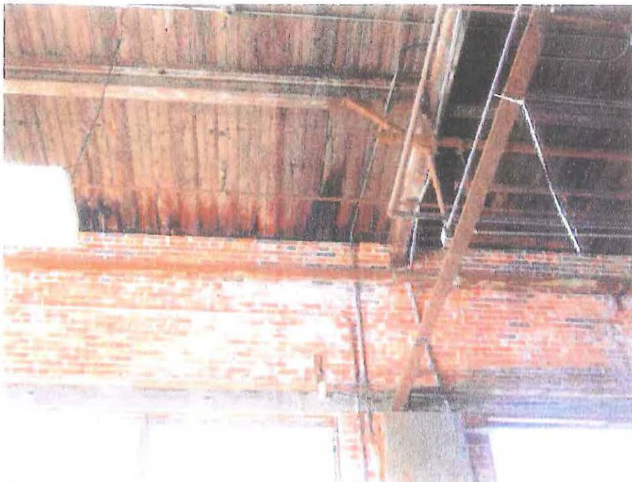
Photo 1-2: Wood deck condition at eave.
