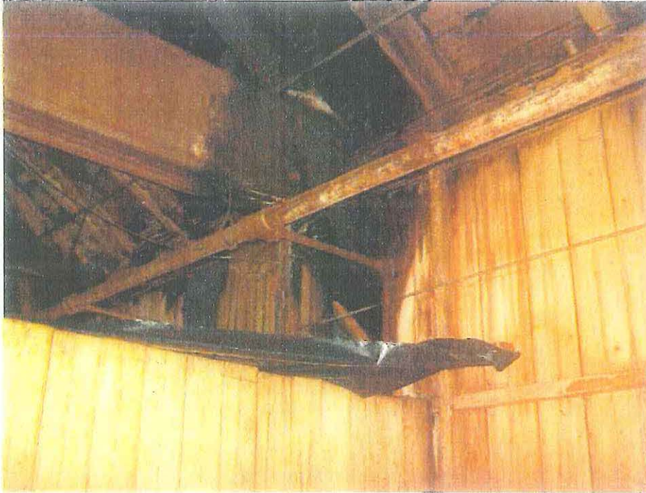
Photo 2-3: Charring of truss top chord.
