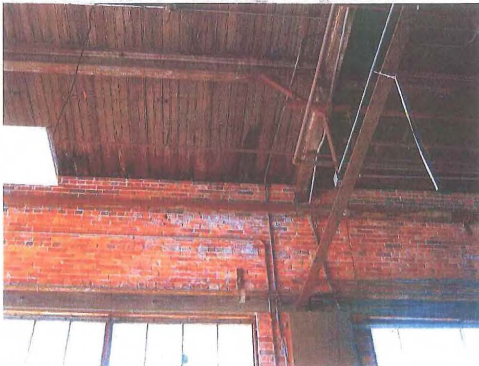
Photo 1-2: Wood deck condition at eave.
