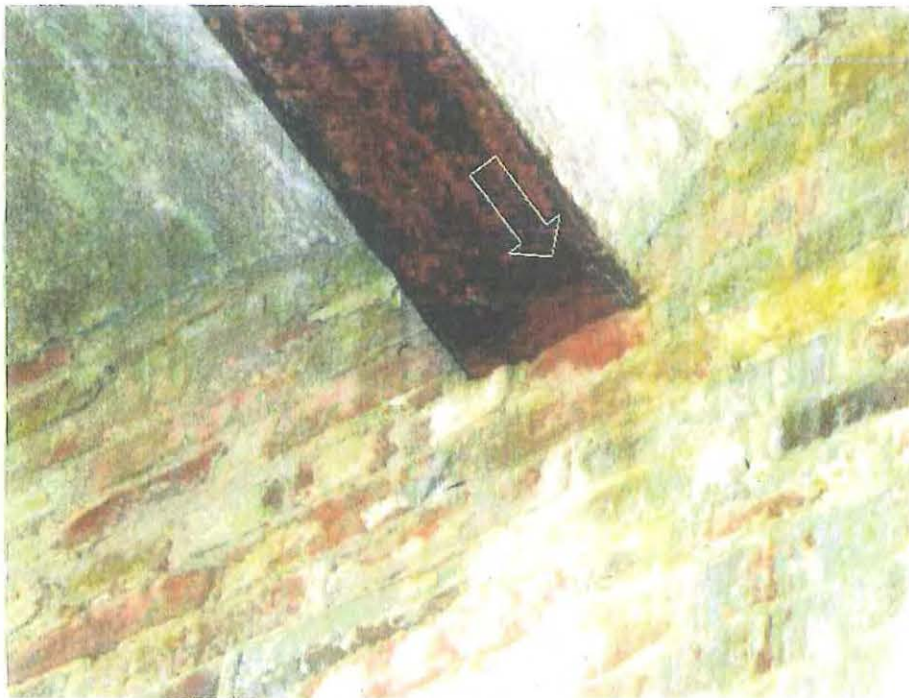
Photo 58-3: Beam end condition with flaking rust.
