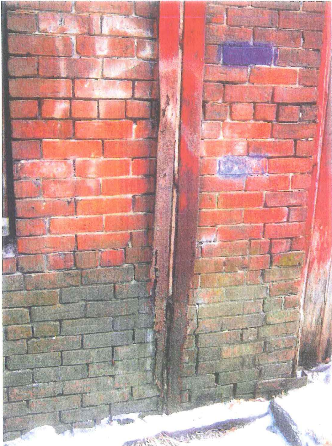
Photo 4-5: Column at exterior wall embedded in masonry. Note column section completely deteriorated. Also note open masonry joints, cracked bricks.
