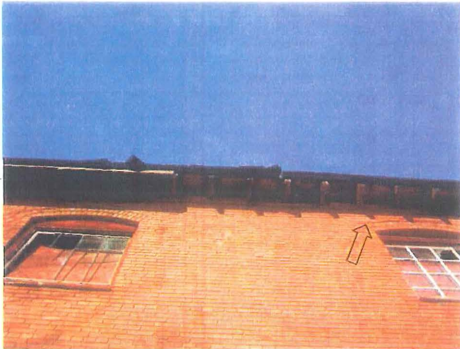
Photo 12-2: Eave with loose slates, missing eave trim, masonry cracking and broken windows.
