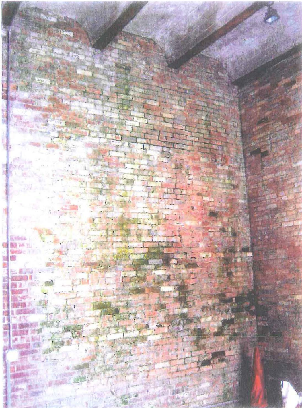
Photo 58-1: Moss growing on interior walls.
