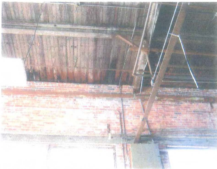
Photo 1-2: Wood deck condition at eave.
