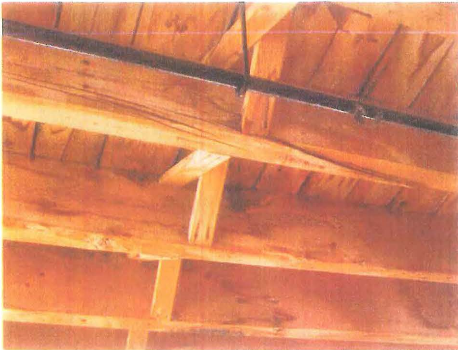
Photo 6A-3: Floor joist splitting.
