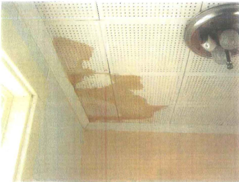
Photo 30-3: Leaking noted at ceiling adjacent to southwest wall.
