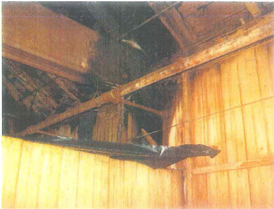
Photo 2-3: Charring of truss top chord.
