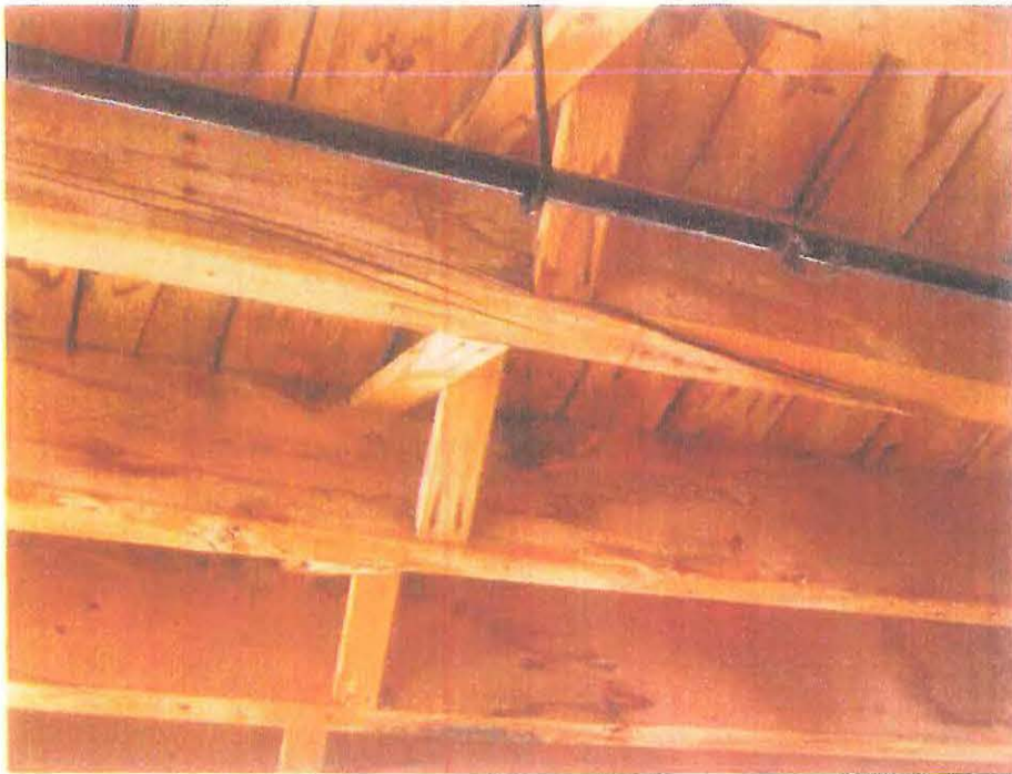
Photo 6A-3: Floor joist splitting.
