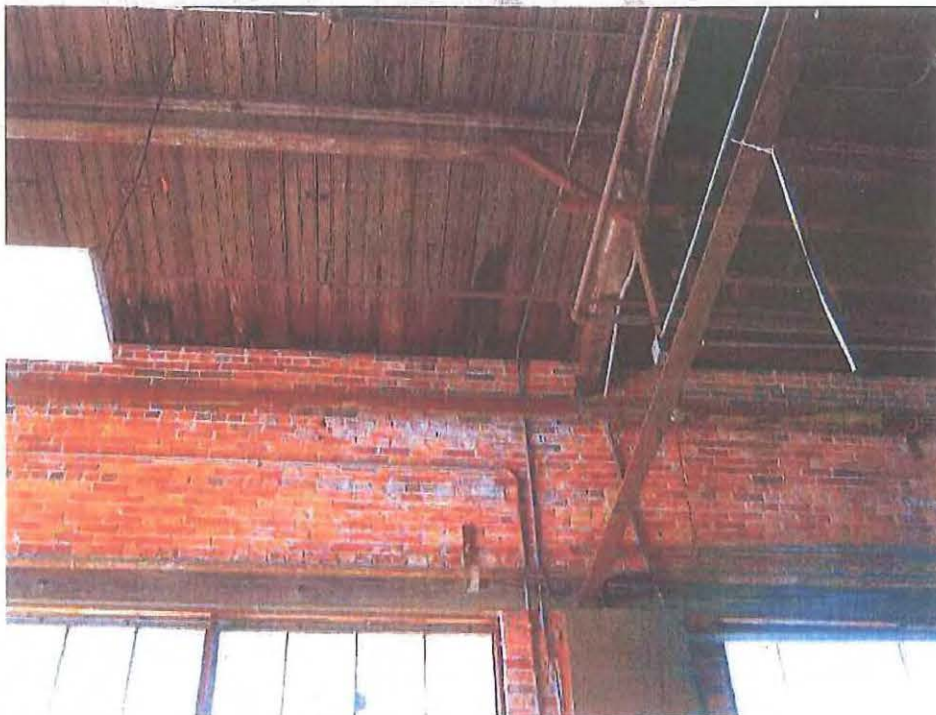
Photo 1-2: Wood deck condition at eave.
