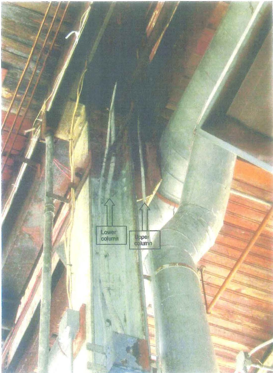
Photo 1-5: Column discontinuity at low-high roof condition.
