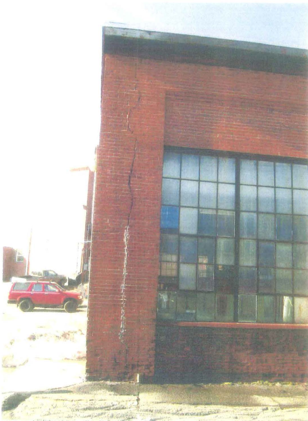
Photo 1-4: Vertical brick masonry crack at southwest pilaster.
