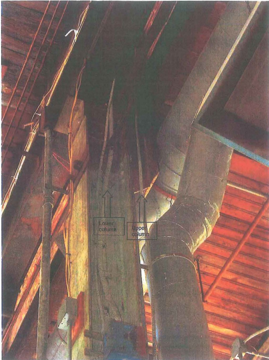
Photo 1-5: Column discontinuity at low-high roof condition.
