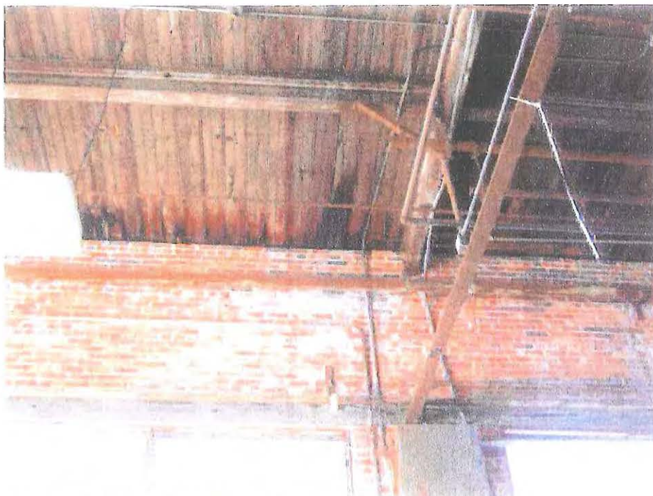
Photo 1-2: Wood deck condition at eave.
