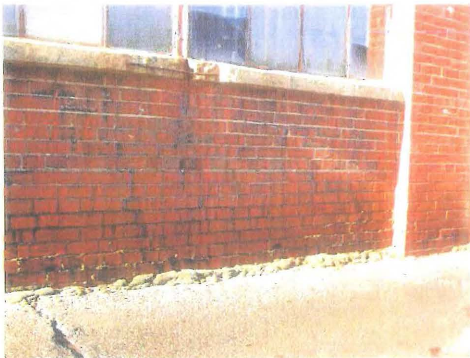
Photo 1-3: Building 1 at eave drip line. Note sill condition, window condition, moss and missing mortar.
