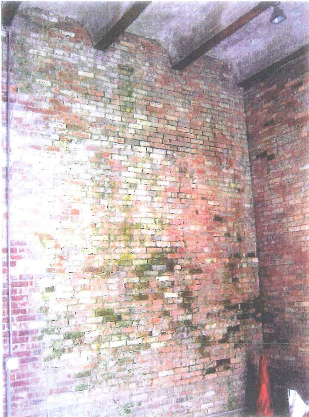
Photo 58-1: Moss growing on interior walls.
