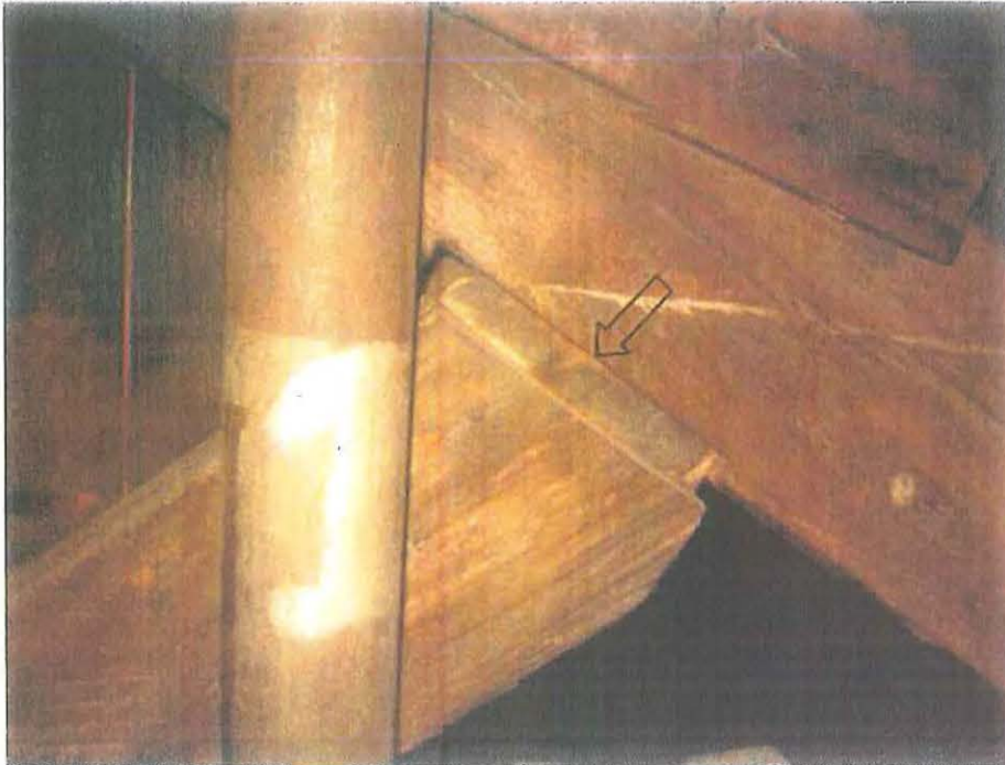
Photo 2-5: Timber truss joint separation.
