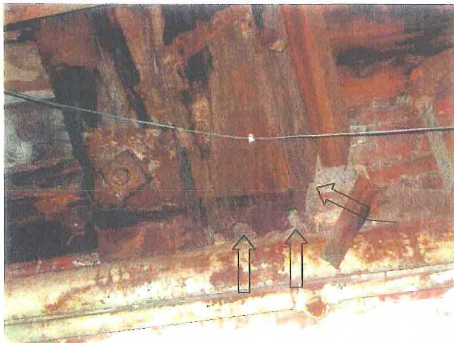
Photo 6B-2: Failed (deteriorated) end of timber truss supporting exterior wall of Building 6A.
