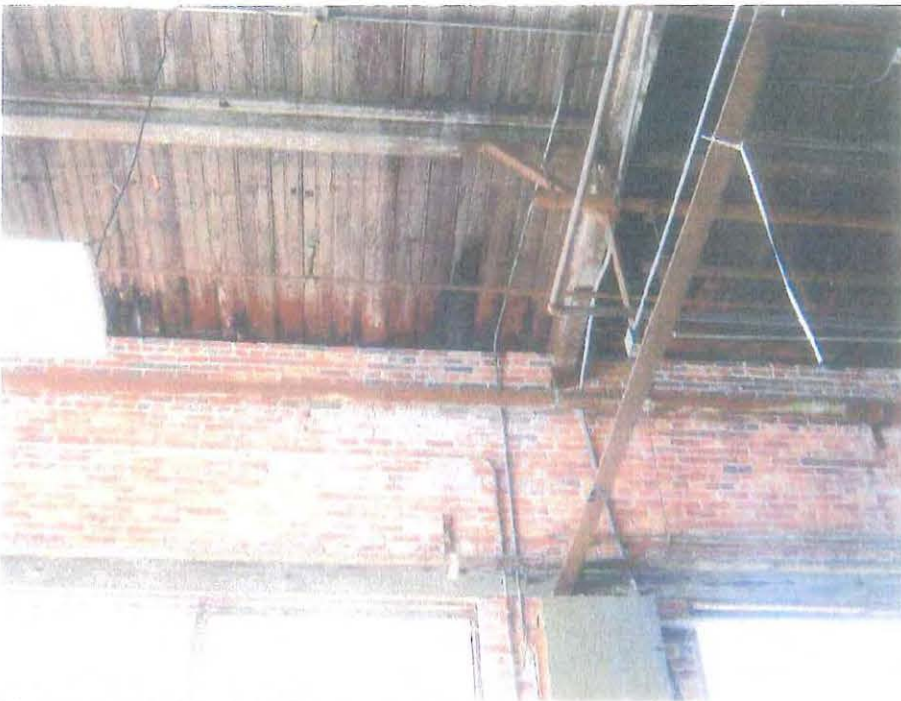
Photo 1-2: Wood deck condition at eave.
