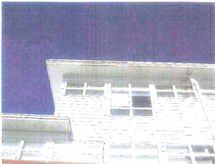
Photo 30-2: Peeling paint at roof eave, uneven siding.
