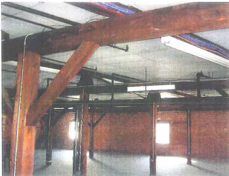
Photo 11-5: Stacked framing system for Building 11 roof. Note leak catch bucket behind column.
