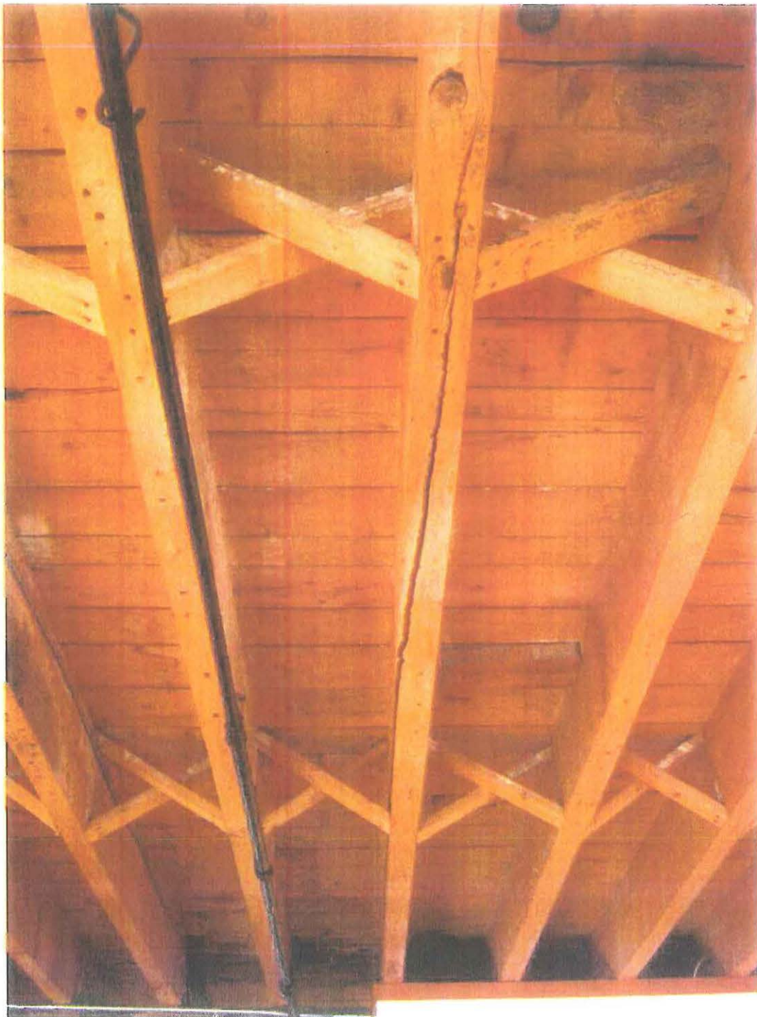
Photo 6A-4: Floor joist splitting.
