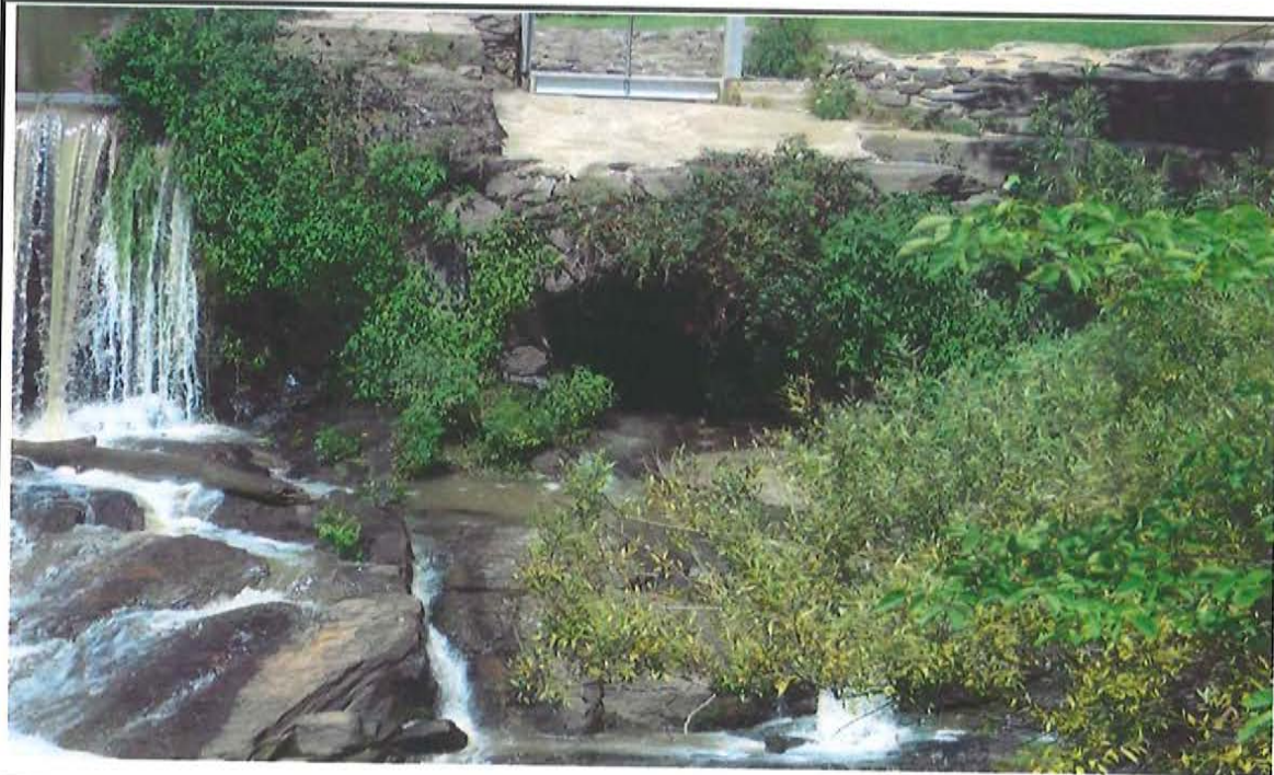
Photo 9 of 24 Looking low-level outlet culvert opening heavy vegetation
