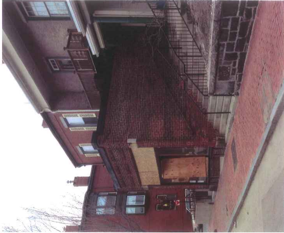
2 Black Painted Heat Pumps
