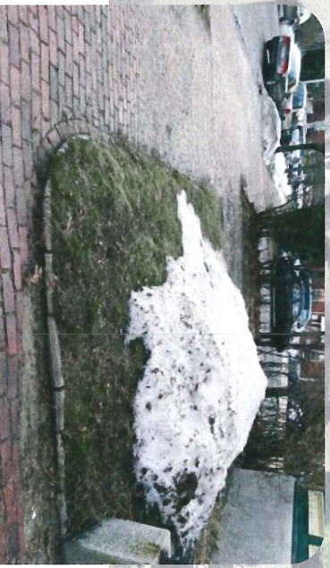
Image 22: Concrete edging 59 Deering Street
