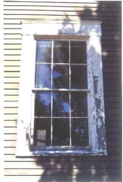
Typical Annex Window
