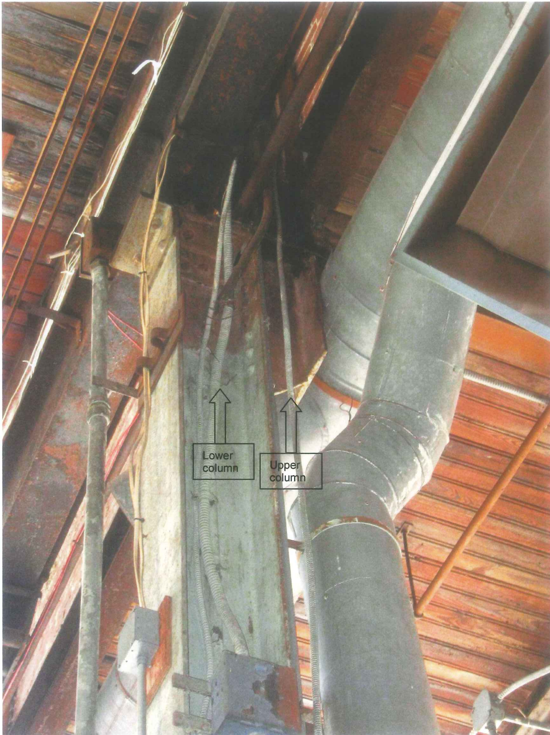
Photo 1-5: Column discontinuity at low-high roof condition.
