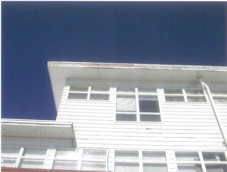
Photo 30-2: Peeling paint at roof eave, uneven siding.
