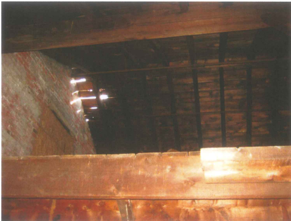
Photo 12-3: Daylight visible at through roof sheathing. Condition is at both ends of roof.
