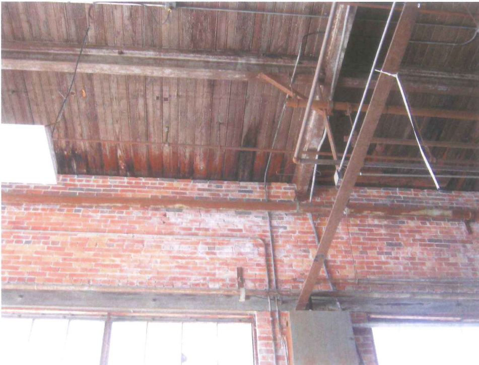
Photo 1-2: Wood deck condition at eave.
