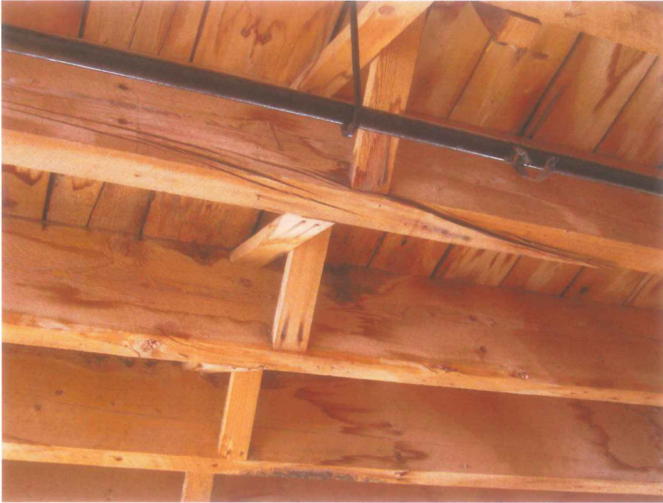
Photo 6A-3: Floor joist splitting.
