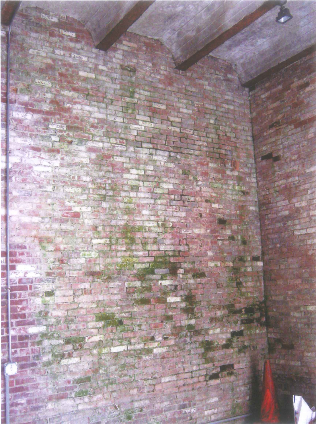
Photo 58-1: Moss growing on interior walls.
