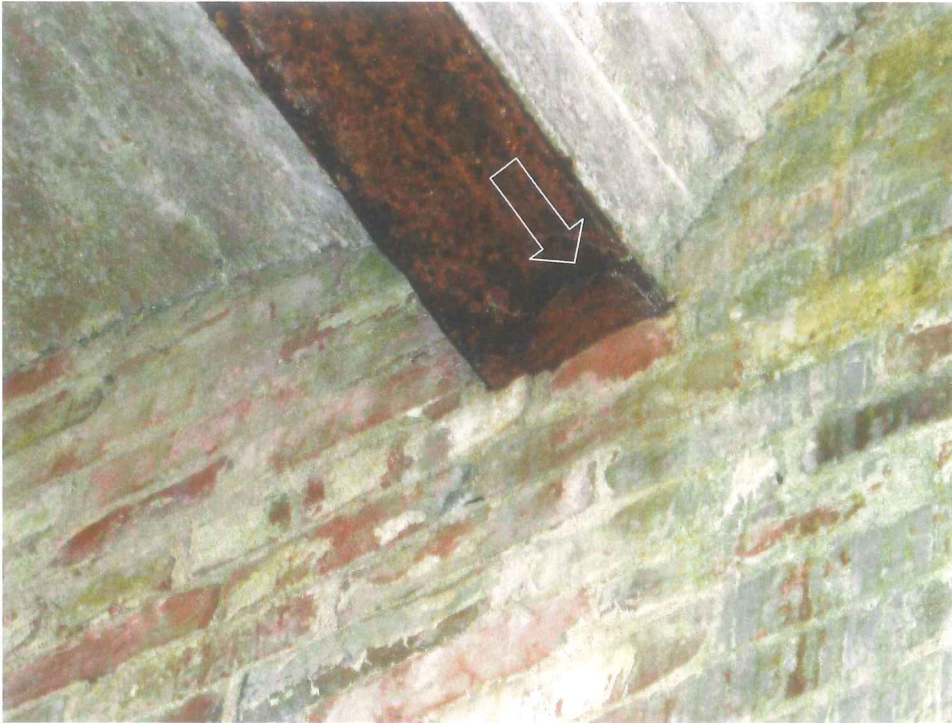
Photo 58-3: Beam end condition with flaking rust.
