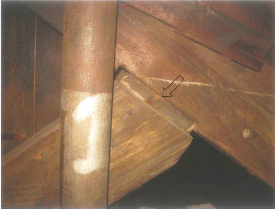
Photo 2-5: Timber truss joint separation.
