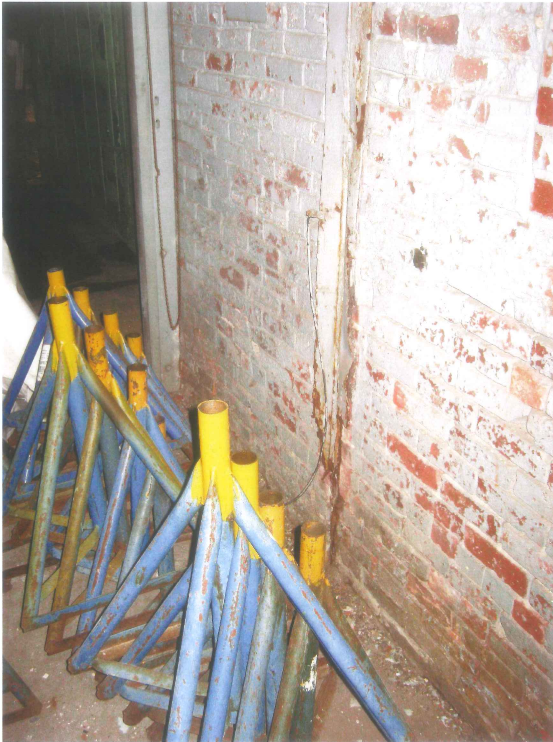
Photo 4-4: Column at exterior wall embedded in masonry. Note column section completely deteriorated.
