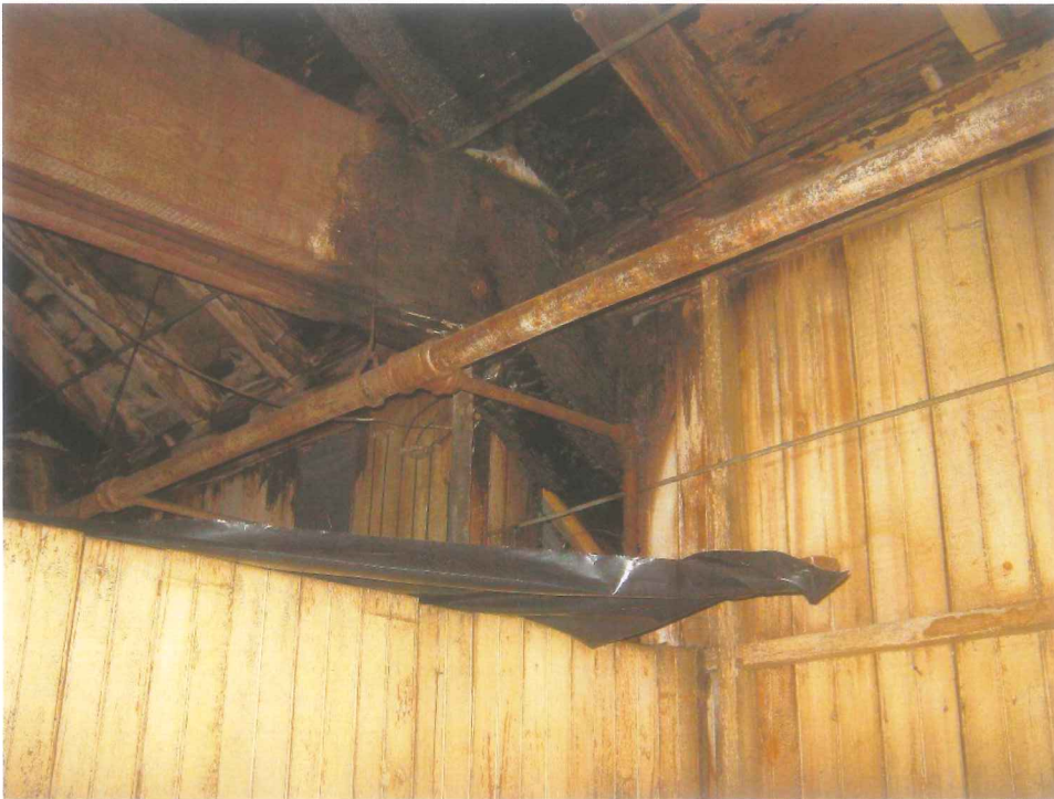
Photo 2-3: Charring of truss top chord.
