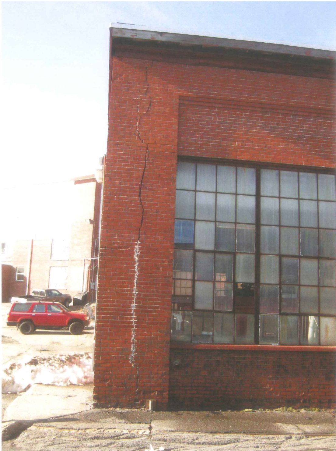
Photo 1-4: Vertical brick masonry crack at southwest pilaster.
