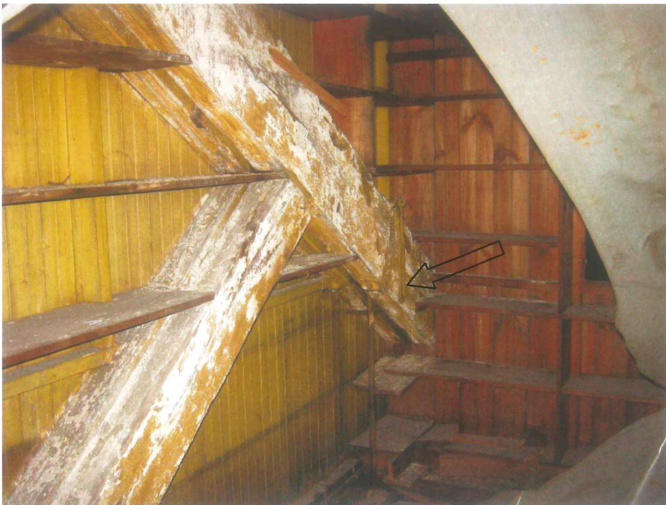
Photo 2-4: Broken truss hanger saddle hanger.
