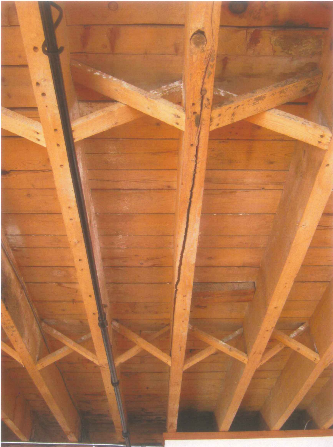
Photo 6A-4: Floor joist splitting.
