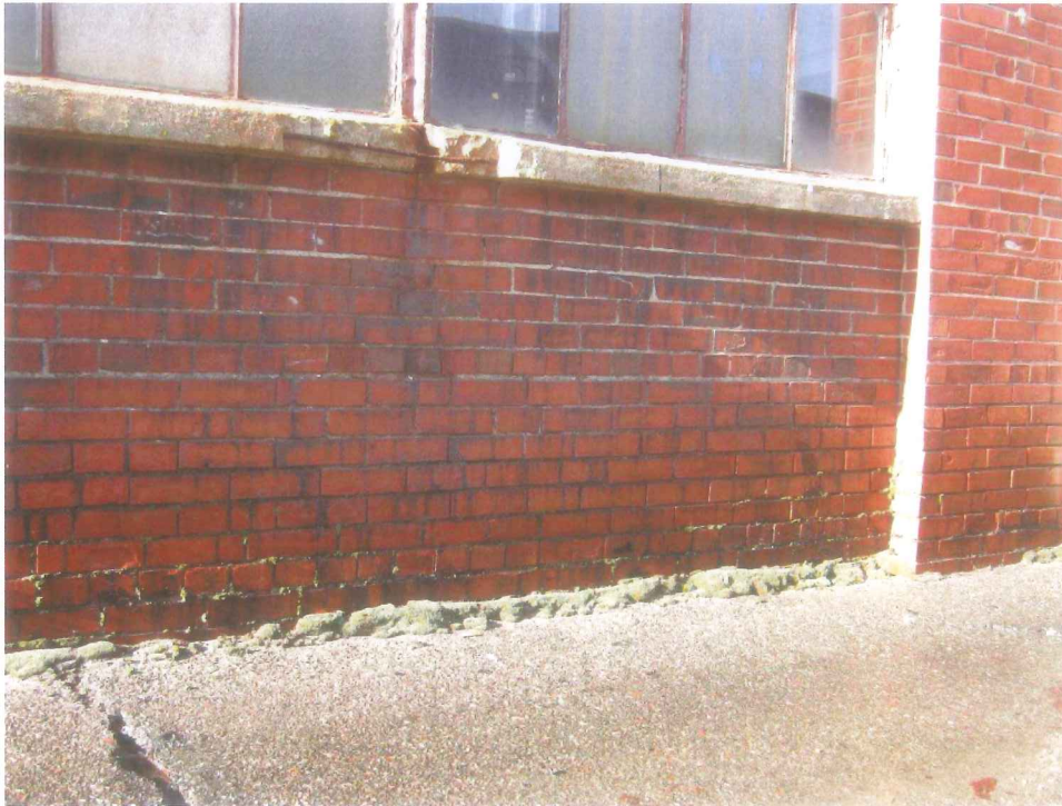
Photo 1-3: Building 1 at eave drip line. Note sill condition, window condition, moss and missing mortar.
