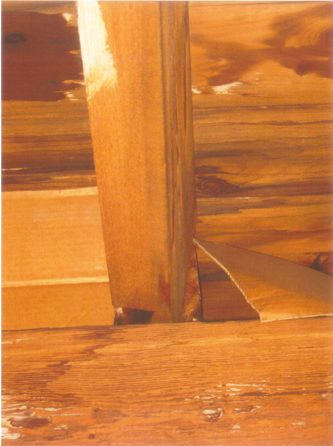
Photo 6A-5: Rotated roof rafter and evidence of prior leaking.
