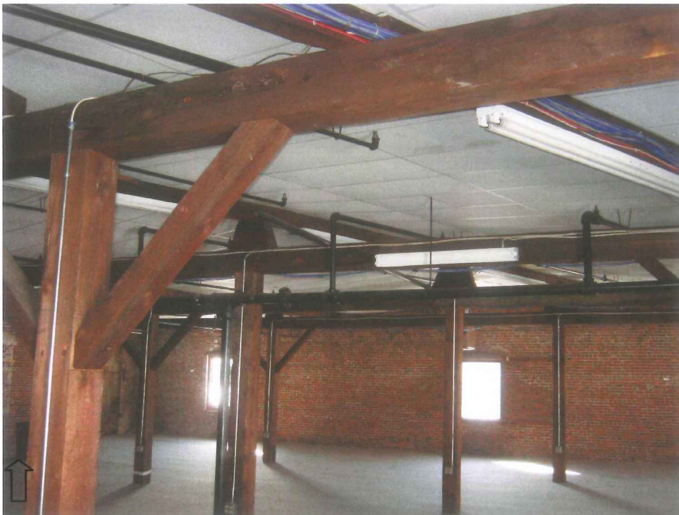
Photo 11-5: Stacked framing system for Building 11 roof. Note leak catch bucket behind column.
