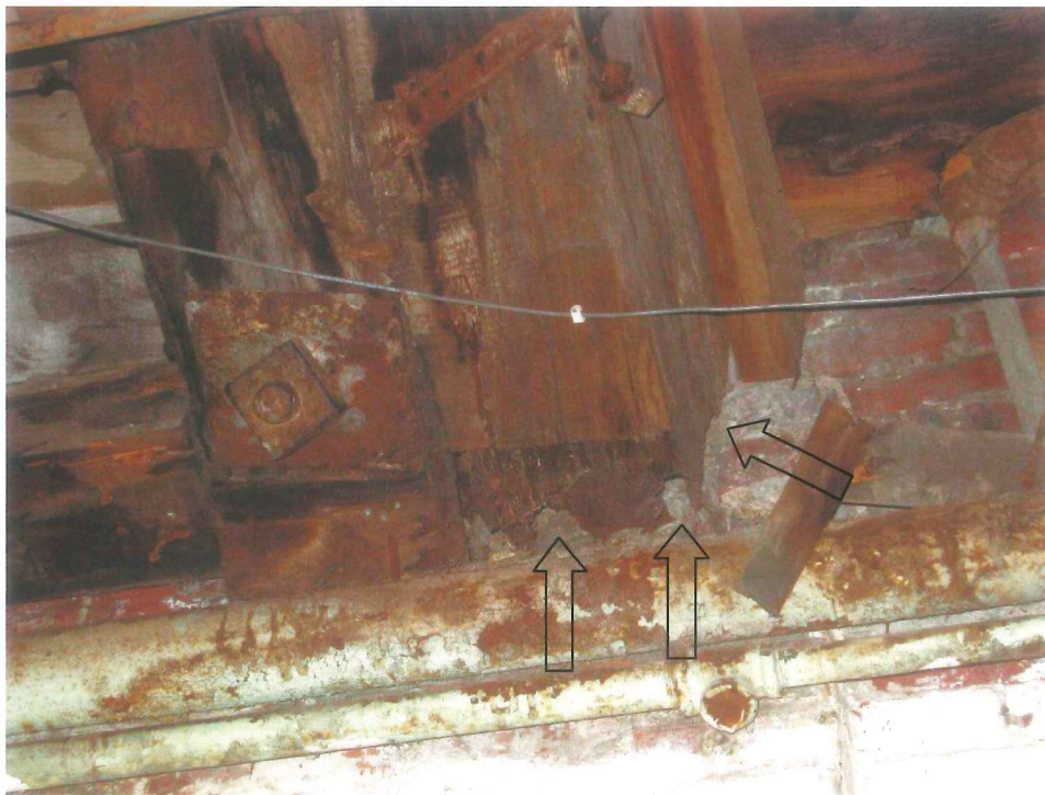
Photo 6B-2: Failed (deteriorated) end of timber truss supporting exterior wall of Building 6A.
