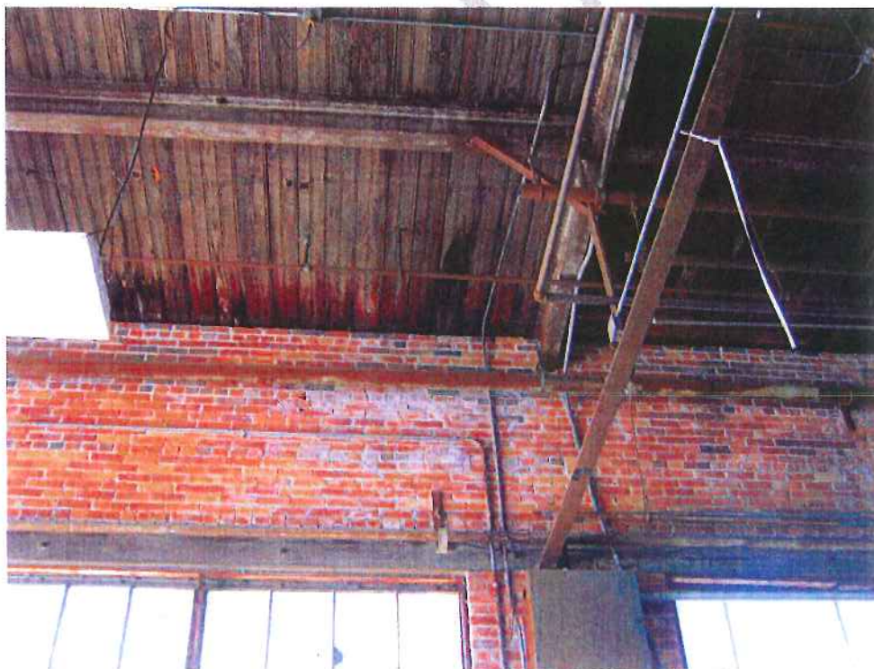
Photo 1-2: Wood deck condition at eave.
