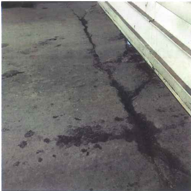
settlement and cracking in conc slab by overhead door
