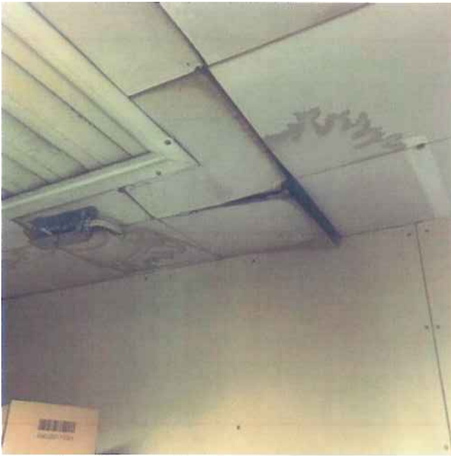
water leak from roof
