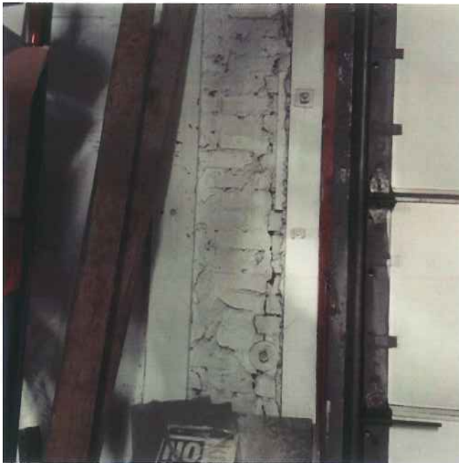
damage to masonry bearing wall at overhead door
