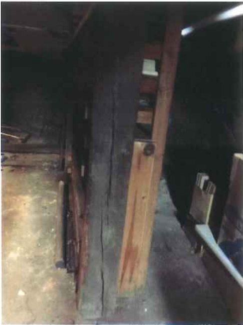
Cracked basement post
