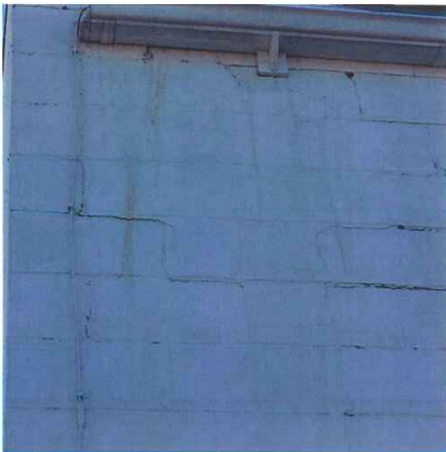
settlement cracks in cmu bearing wall
