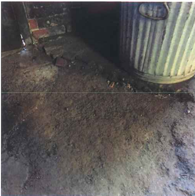
differential settlement and cracking of slab
