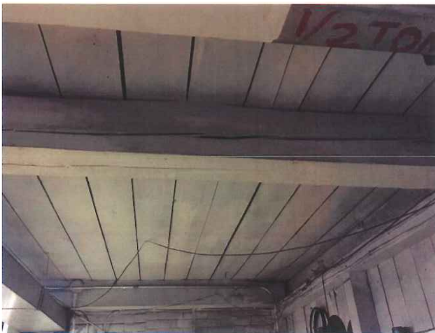
severely checked wood beam
