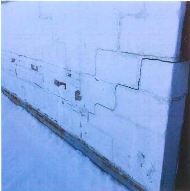
severely compromised cmu bearing wall with complete horizontal thru crack
