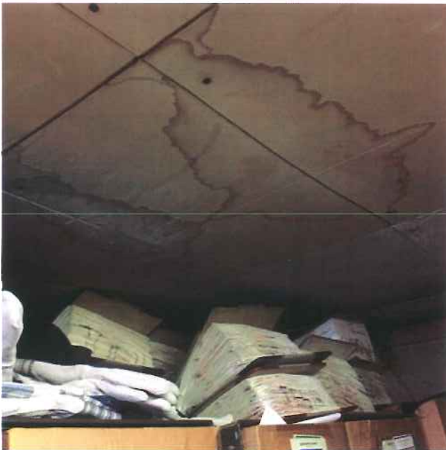
water leak at front building second floor office roof
