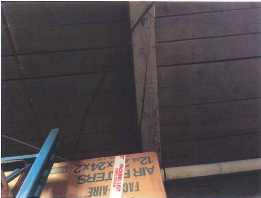
completely cracked roof beam. Total failure of member
