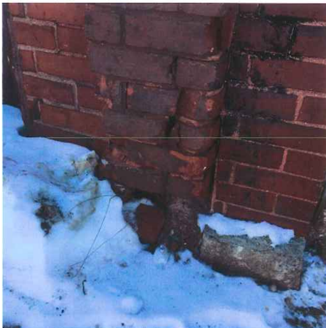
deteriorated brick masonry bearing wall
