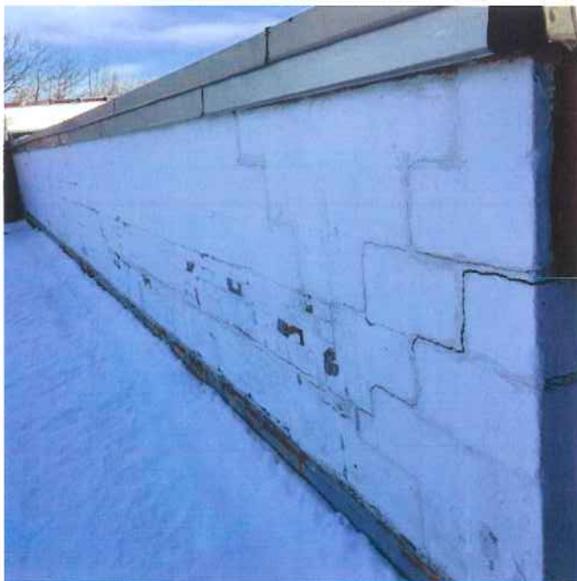
severe horizontal crack runs full length of wall
