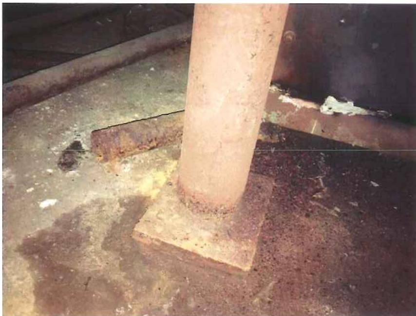
corroded basement support post
