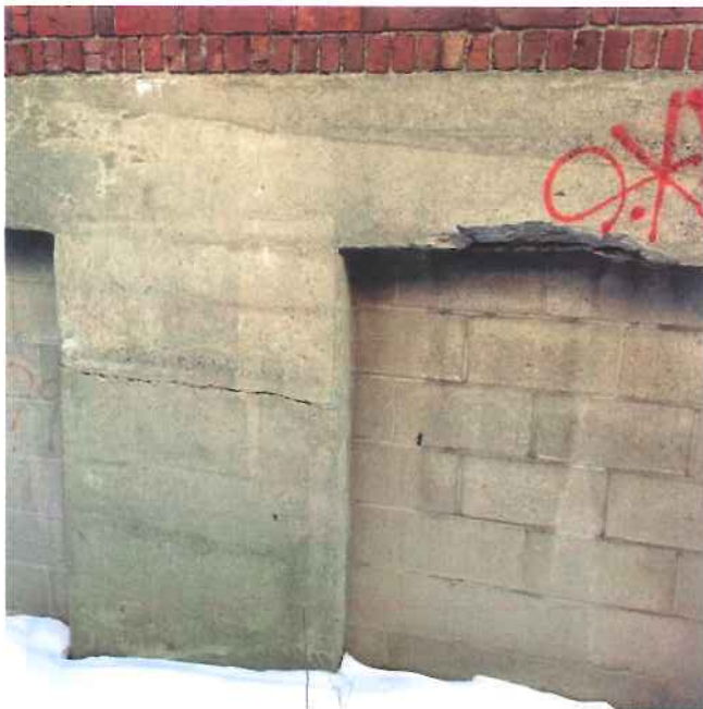
foundation wall thru crack
