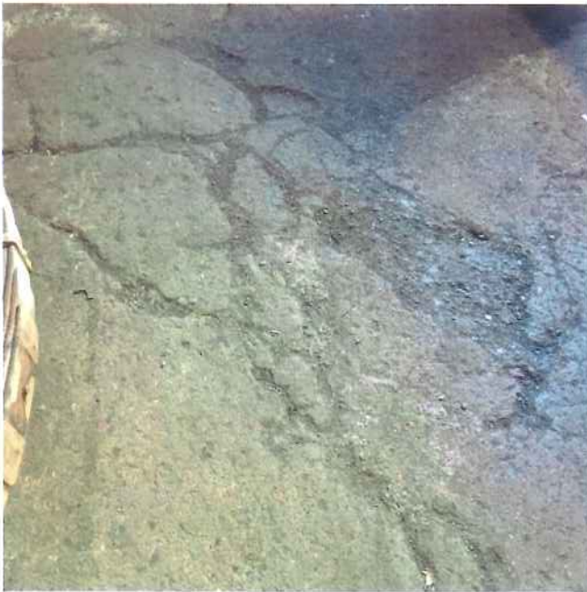
wear and cracking in conc. slab
