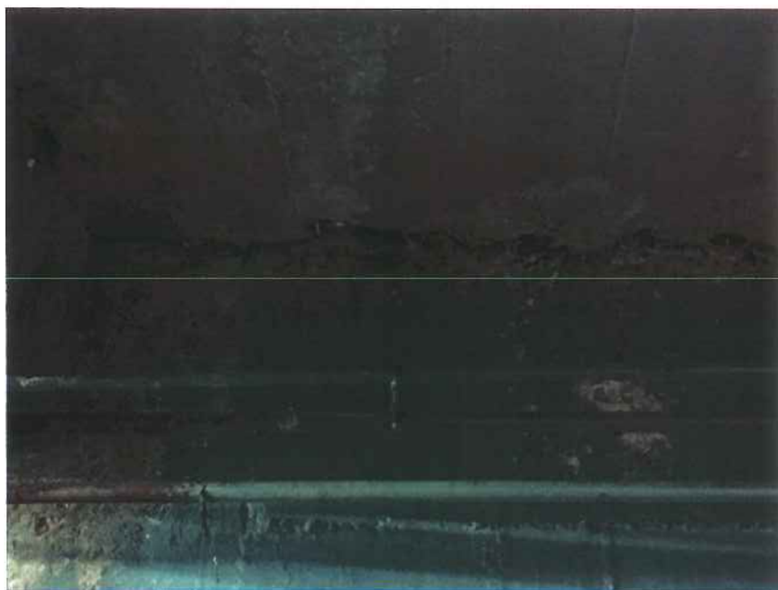
severe degradation at floor/wall connection
