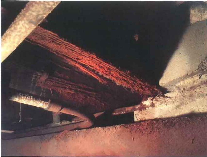
severely deteriorated floor joist at first floor framing
