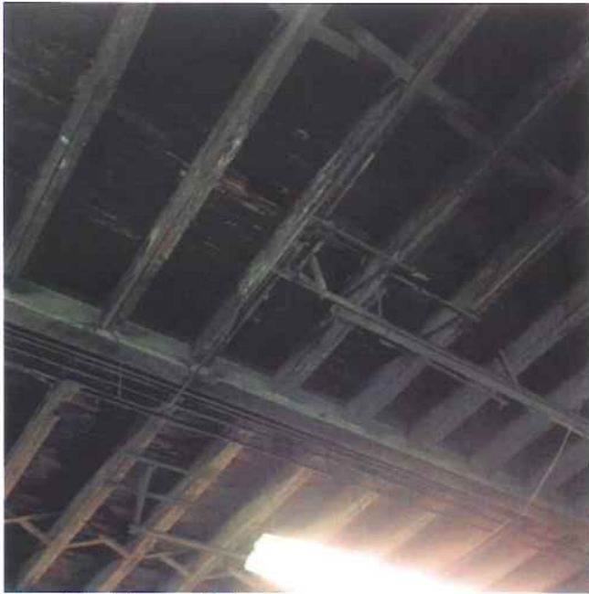
rotted leaking roof decking
