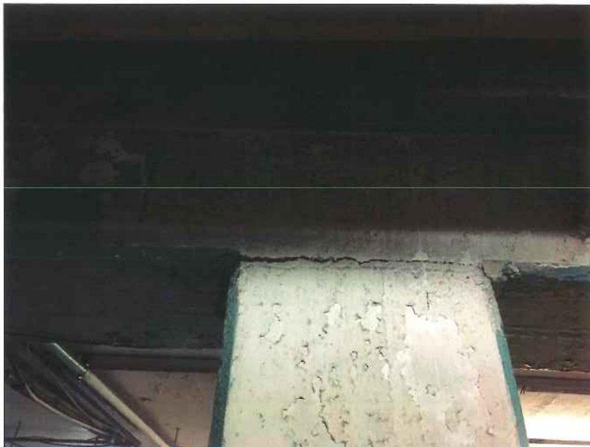
catastrophic thru crack at beam/column connection
