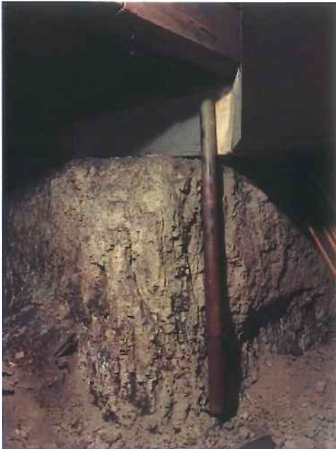
Corroded detached steel post clay soil behind.
