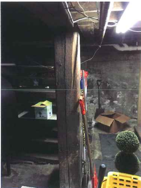
Cracked post and support beam
