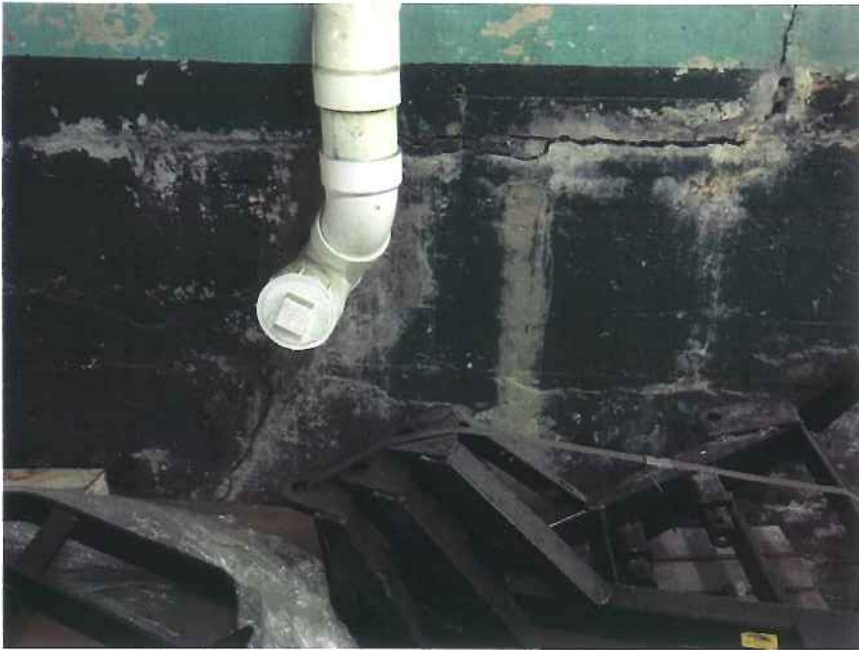
severe cracking in foundation wall
