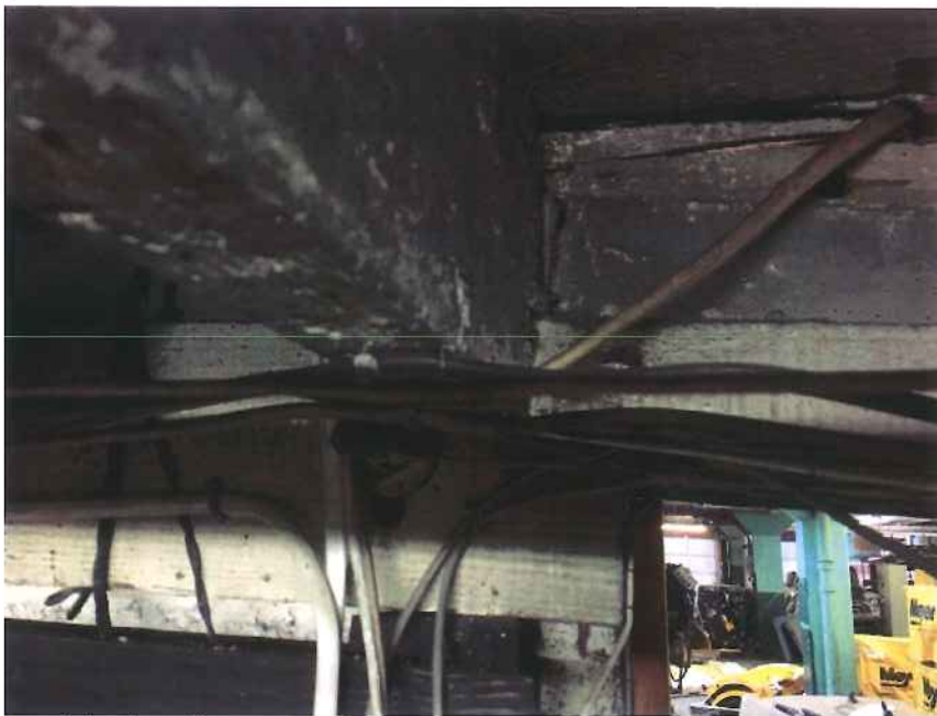
crack in first floor support beam
