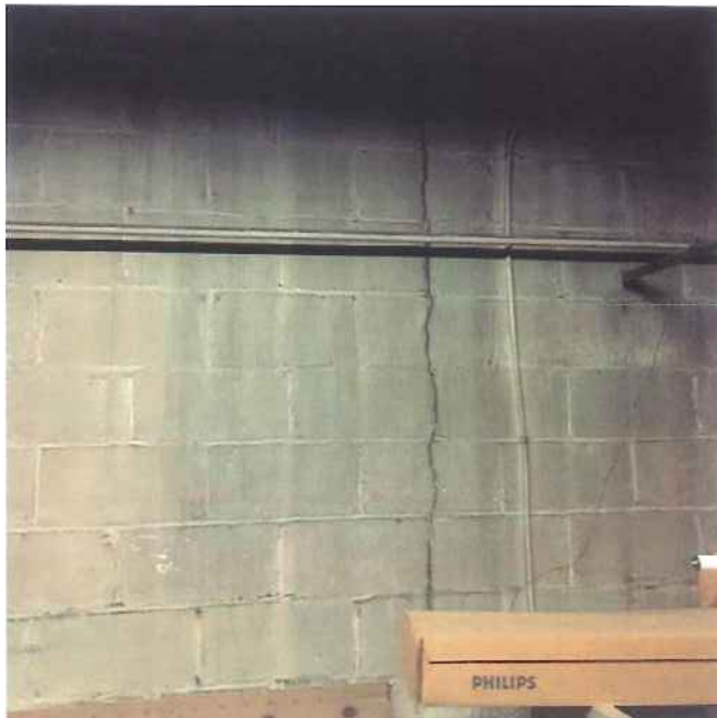
vertical wall crack in load bearing cmu at newer addition
