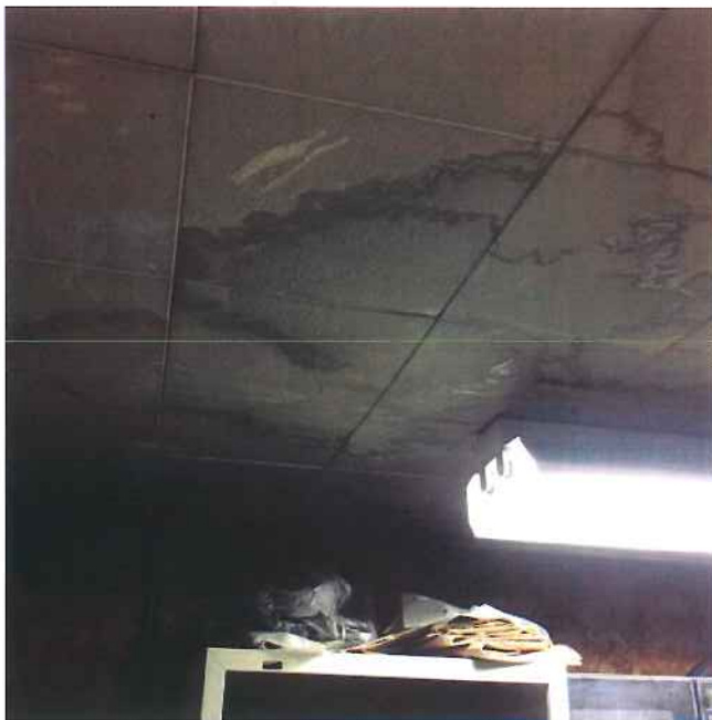
water stain due to roof leak at rotted decking
