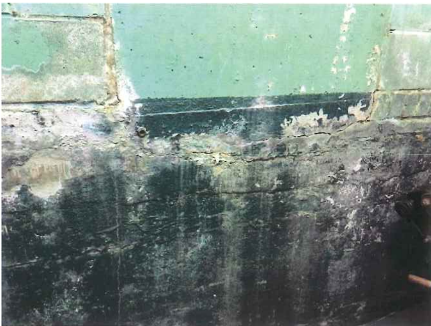
severe cracking in foundation wall
