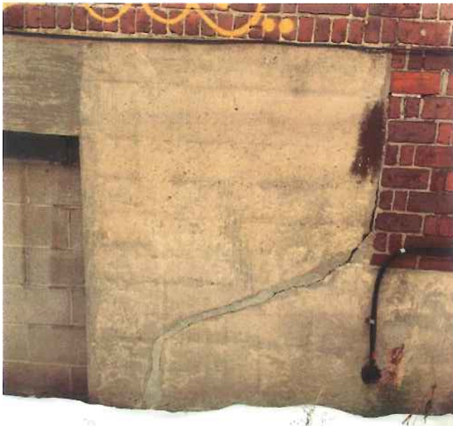
foundation wall damage
