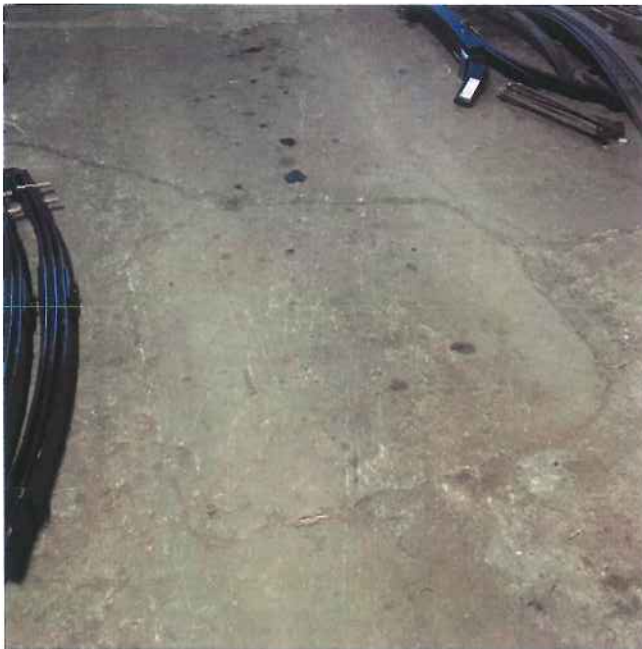
conc slab differential settling and cracks
