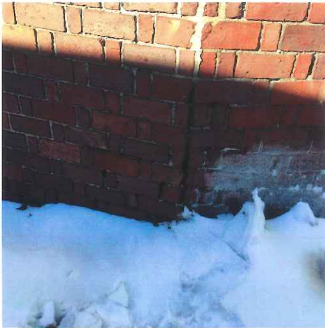
opened masonry joint leaking water into building
