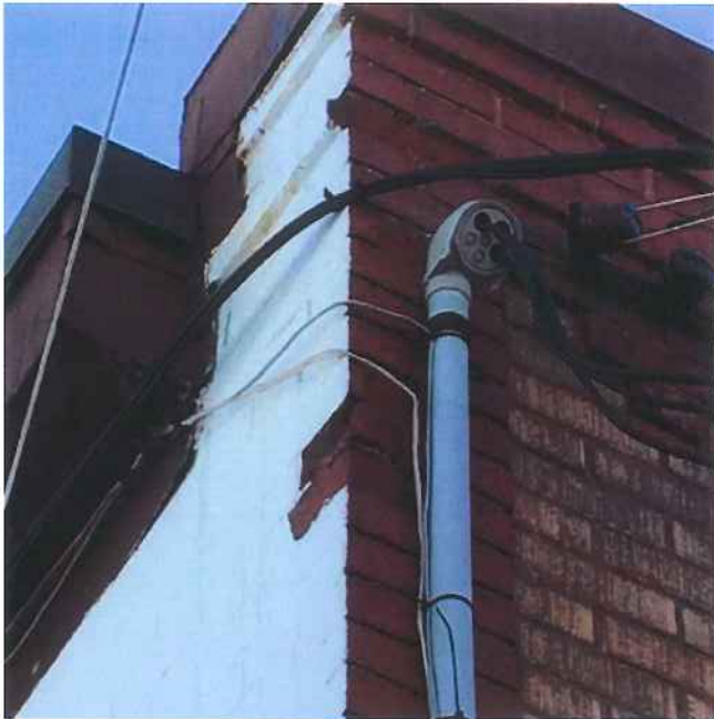
spalled brick face at front of building.
