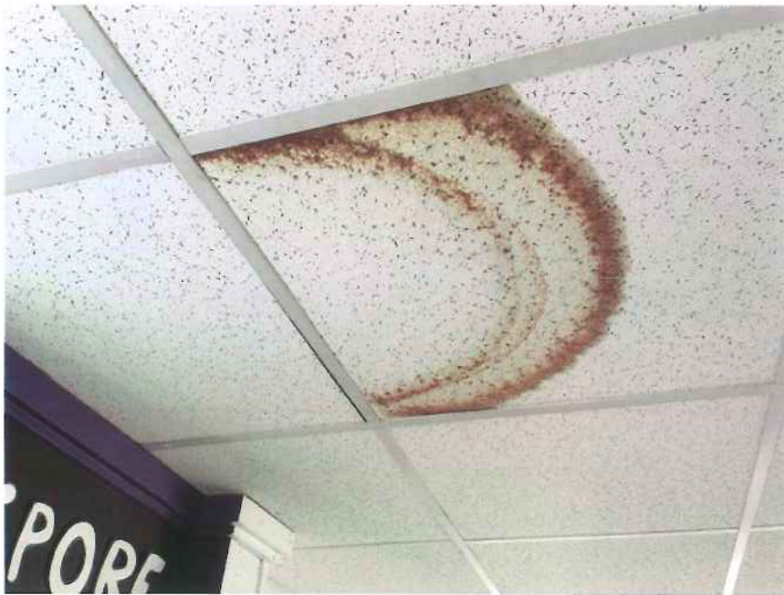
water stain at roof leak
