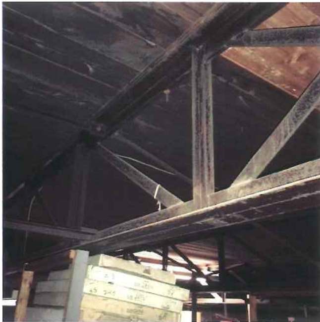
steel bar joist roof framing at newer addition. some roof decking boards replaced. several leaks and deteriorated decking areas.
