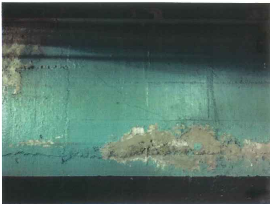
shear crack in concrete beam
