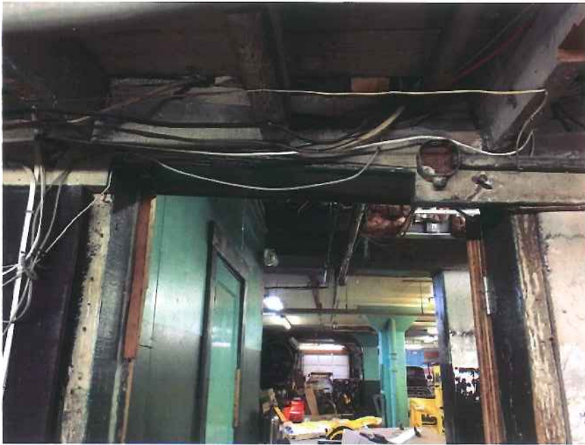
framing failure over door
