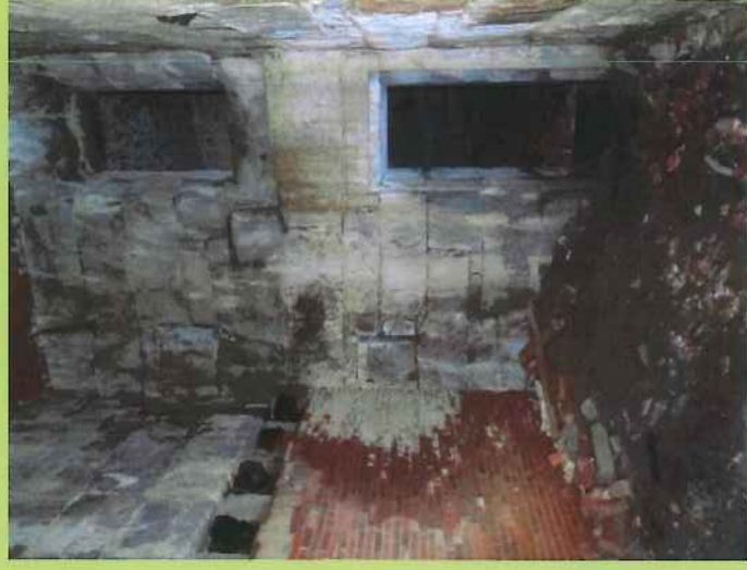
Missing or failing floors
