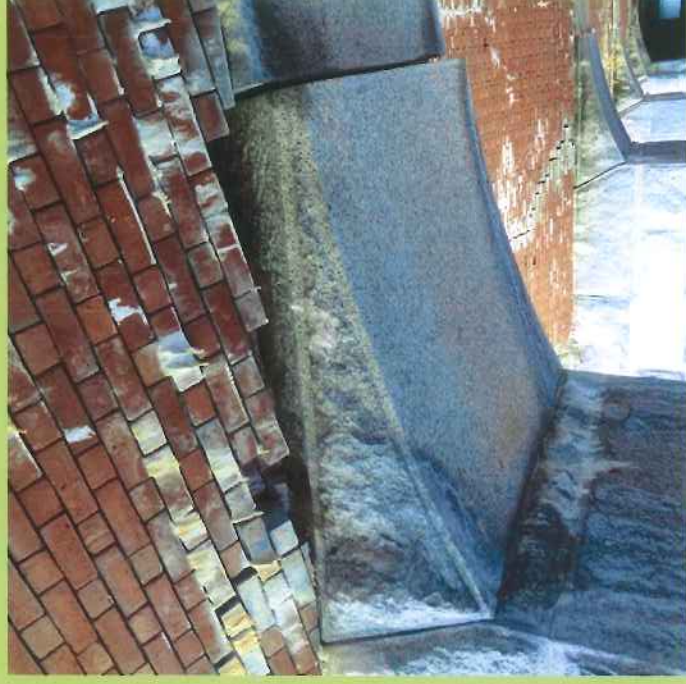
Structural issues with arches
