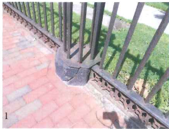
1 Fence needs restoration. Brick sidewalk too high along southern edge
