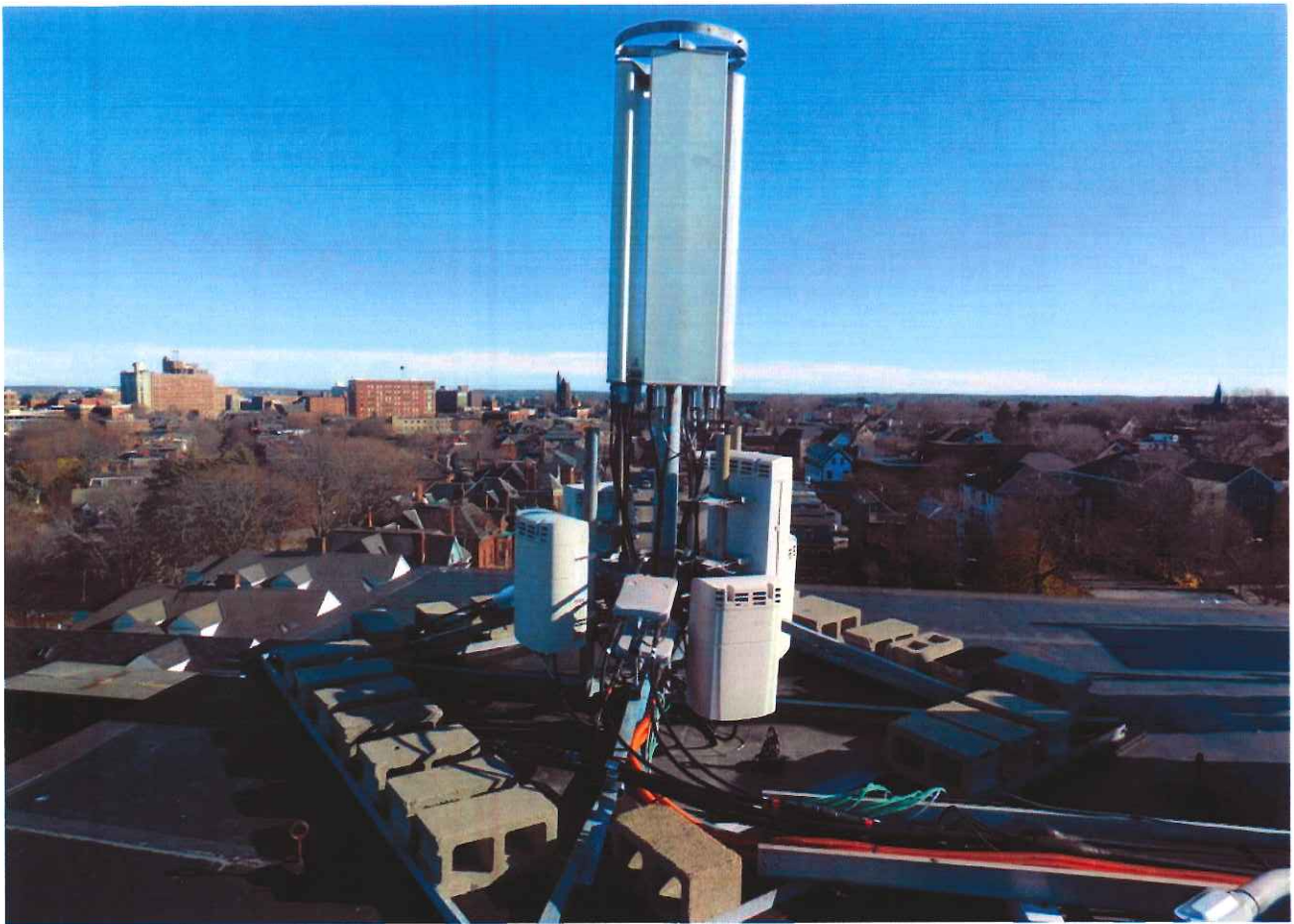
Existing T-Mobile Ballast Frame on Roof
