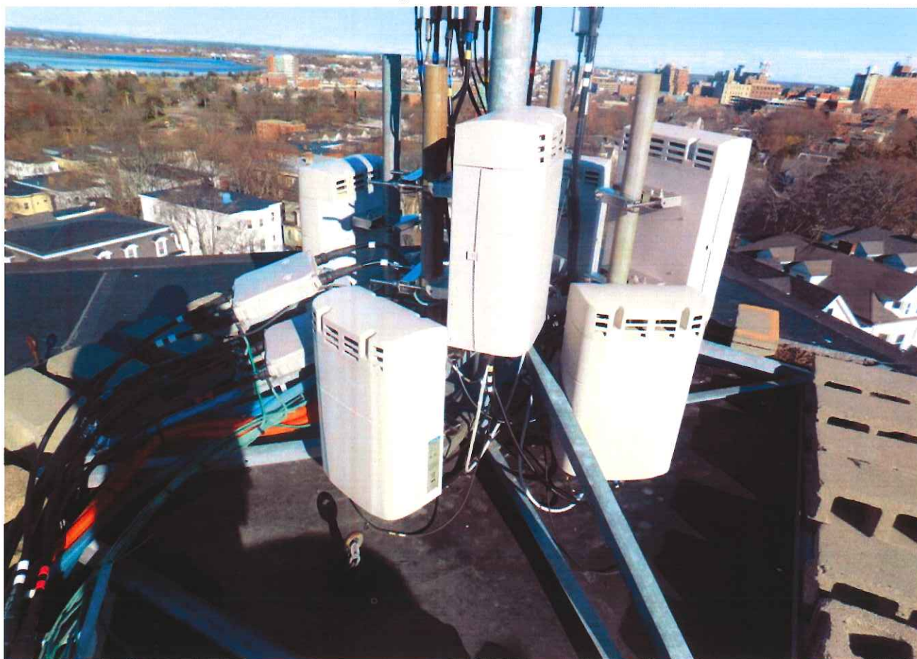
Existing T-Mobile RRH's
